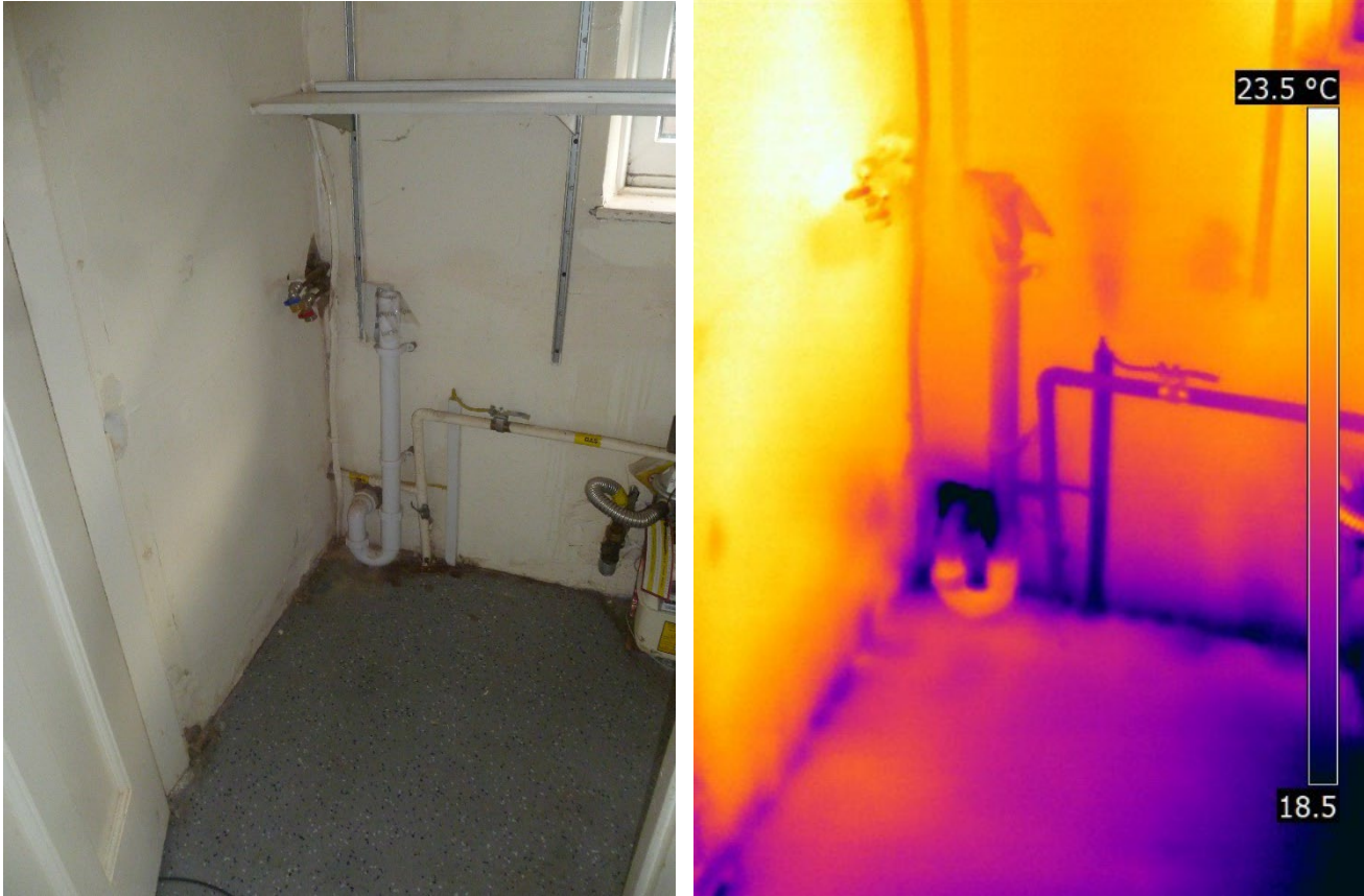
Figure 3-3 Unsealed penetrations in the understairs cupboard in 55AD
