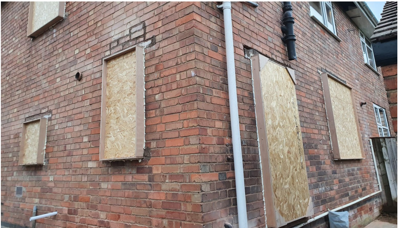
Figure 3-32 Plywood boxes in 55AD to accommodate new external windows and doors in-line with the proposed EWI
