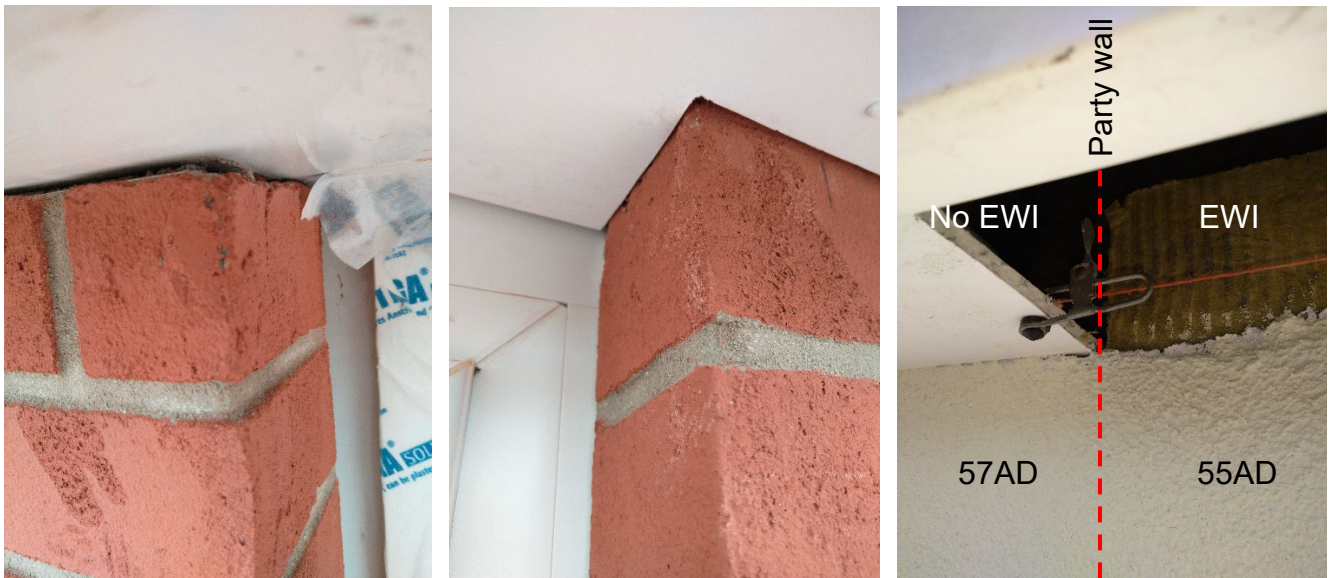
Figure 3-27 EWI stops at soffit level in 57AD (left) but continues behind soffit in 55AD (centre); view behind the soffit (right) at the party wall showing EWI on 55AD eaves but not 57AD
