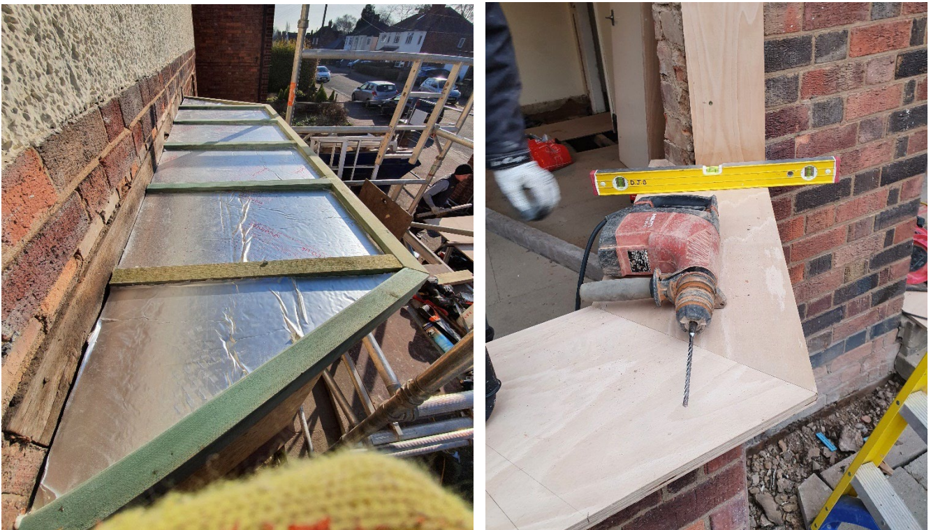
Figure 3-31 Bay roof insulated in 55AD (left) and bay walls and sills extended to accommodate new windows in-line with EWI (right)
