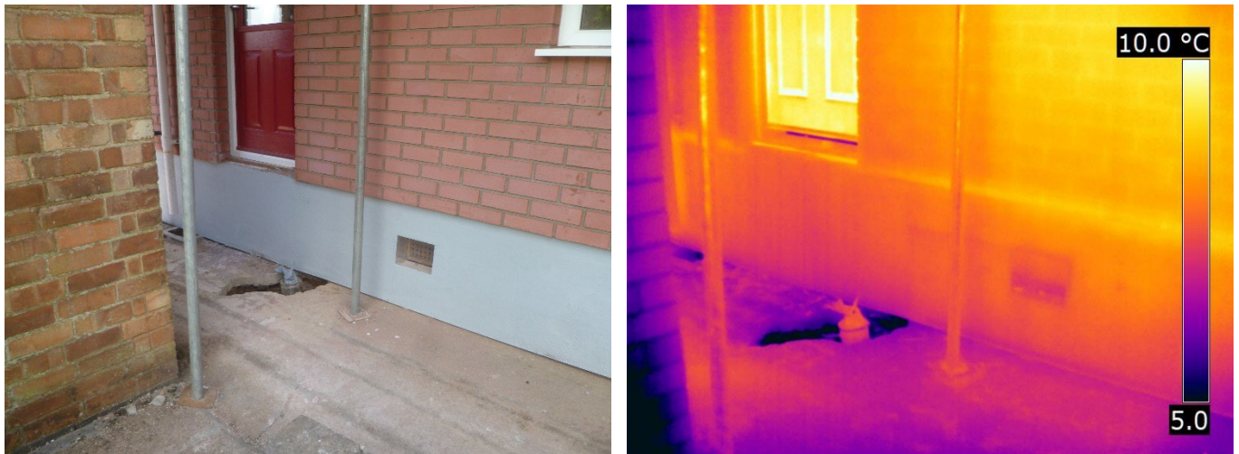
Figure 3-35 XPS insulation below DPC requiring drainage to be relocated underground
