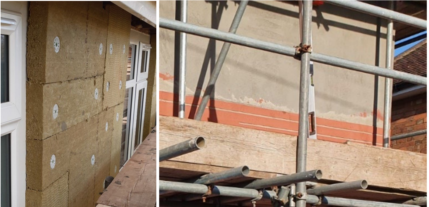
Figure 3-26 Mechanical fixing to wood fibre EWI board (left) followed by render (right)
