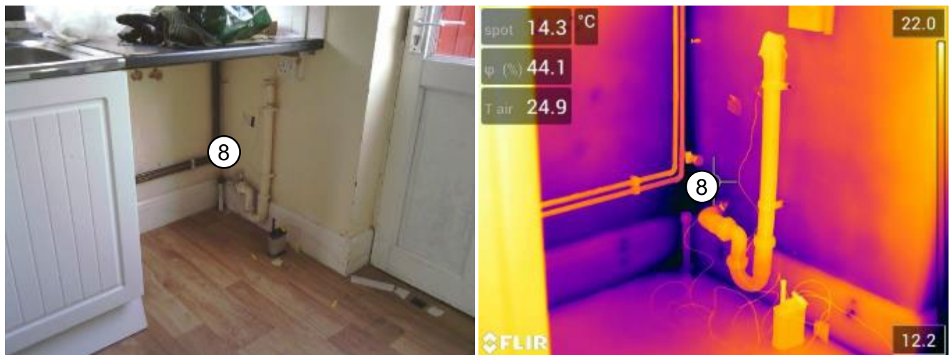
Figure 3-63: External wall waste water pipe penetration (8) thermocouple sensor location.
