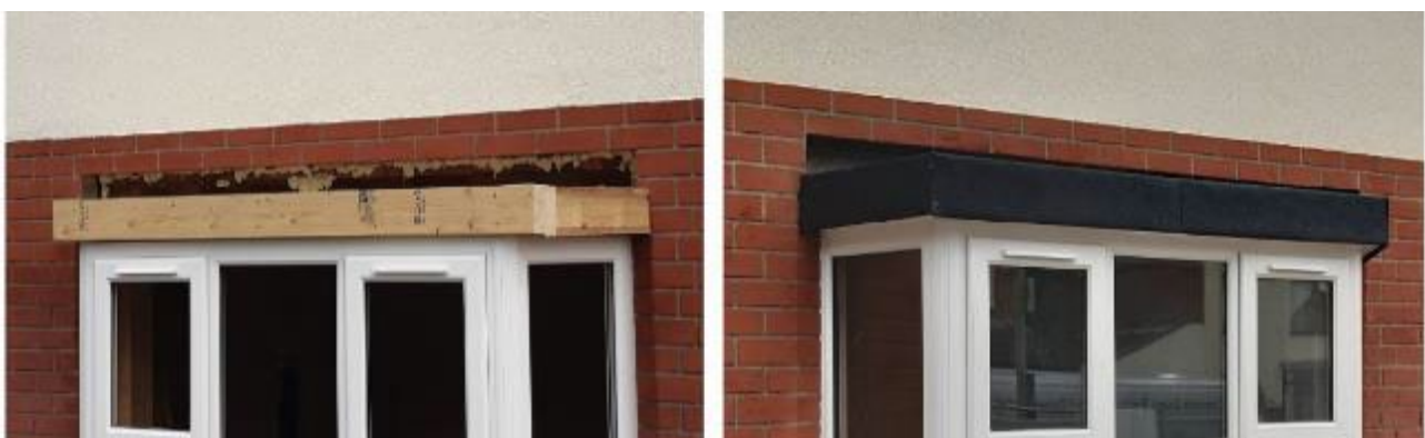
Figure 3-40 Bay window of 57AD being replaced before handover (left) and completed bay window roof of 55AD (right) both showing the large gap between roof and underside of EWI
