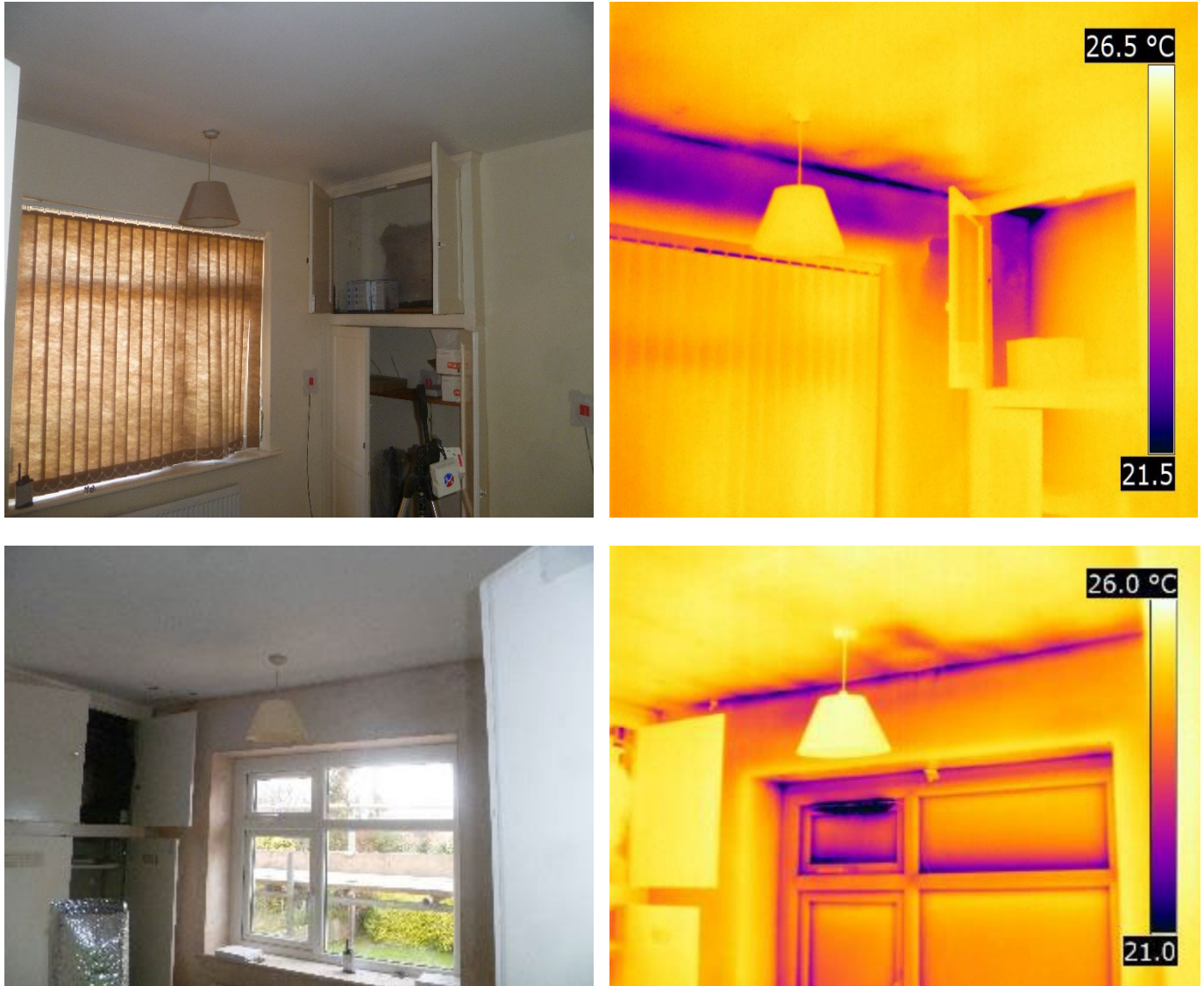
Figure 3-28 Top: thermal bridge at eaves in 57AD where EWI is not installed behind the soffit Bottom: equivalent view in 55AD, with EWI behind the soffit
