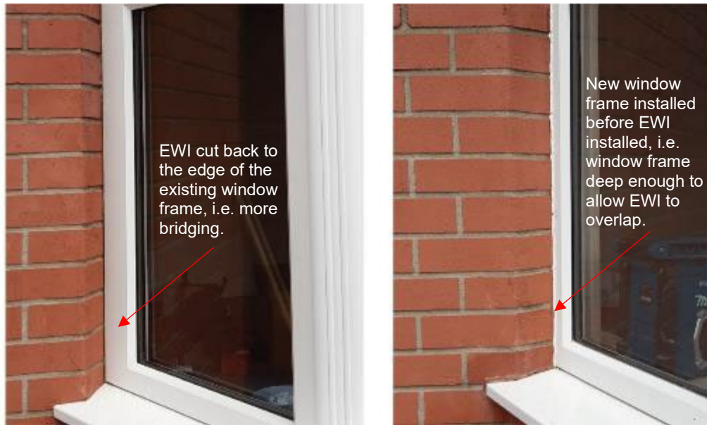
Figure 3-37 57AD bay window (left) where EWI has been cut back in anticipation of a new window, and 55AD bay window (right) where the EWI overlaps the side of the window frame
