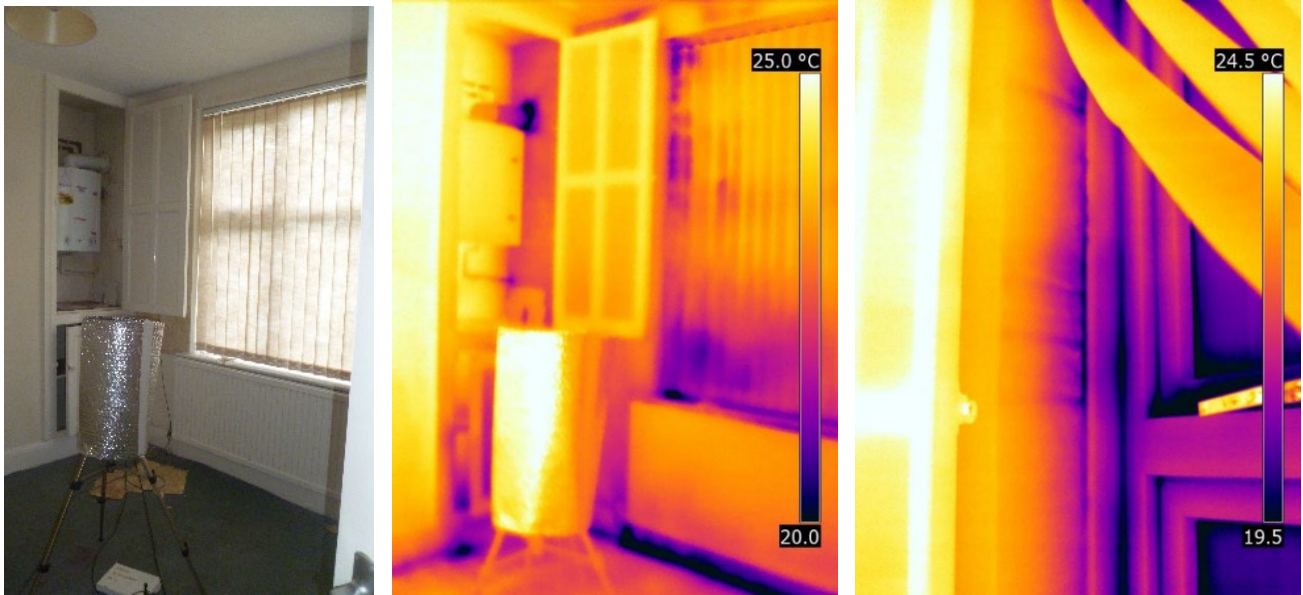
Figure 3-5 Air leakage under depressurisation at ground floor perimeter, cupboard floor, boiler flue and window in 55AD
