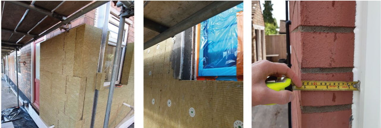
Figure 1-7 Existing windows and doors (not relaced) when EWI installed (57AD); also showing DPC EWI applied to door threshold
