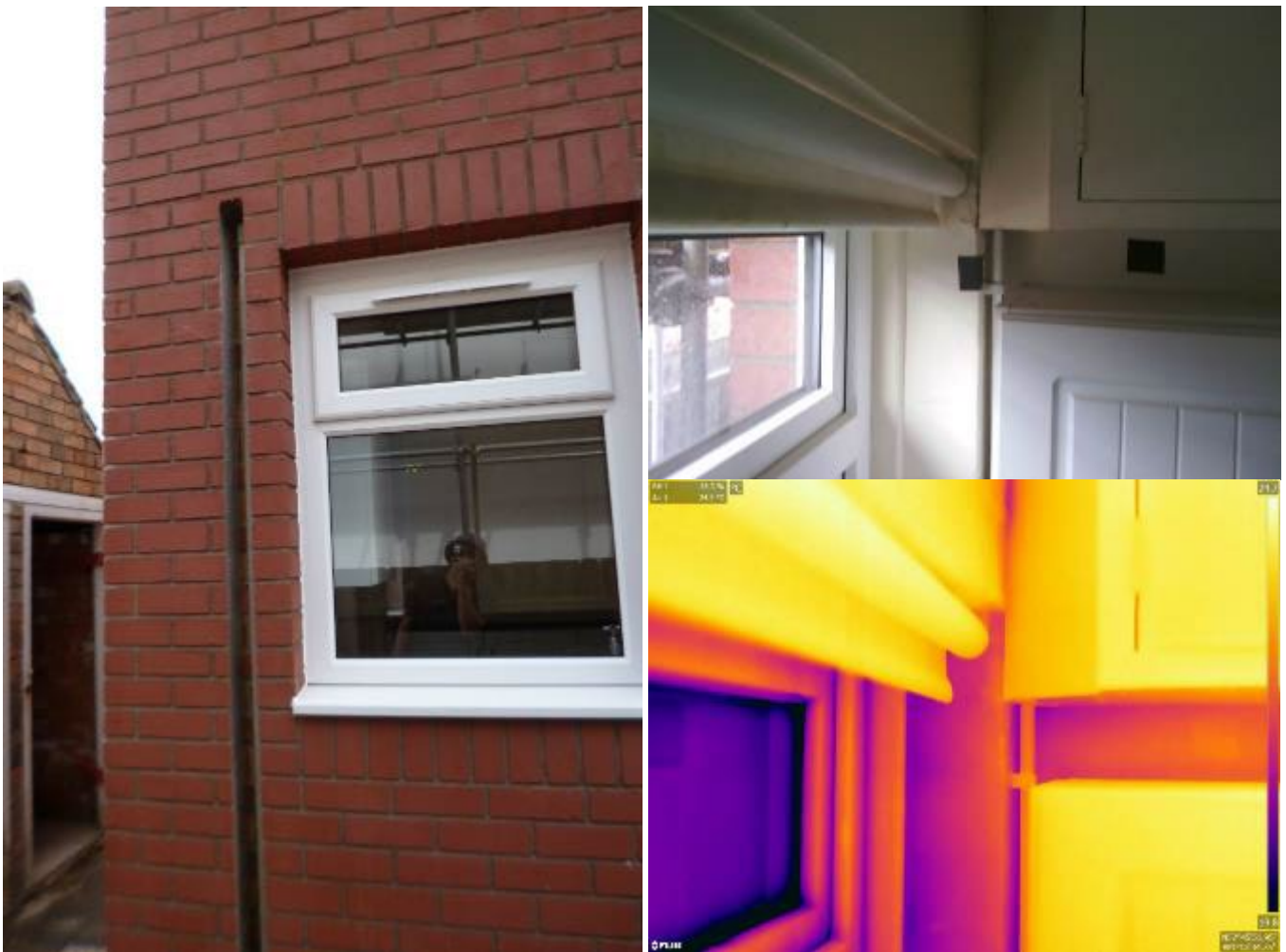
Figure 3-68 Left: 57AD external gas pipe cut-out. Right: internal side of gas pipe cut-out.
