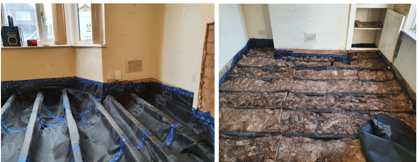
Figure 3-33 Ground floor retrofit with air barrier membrane (left) and mineral wool (right)
