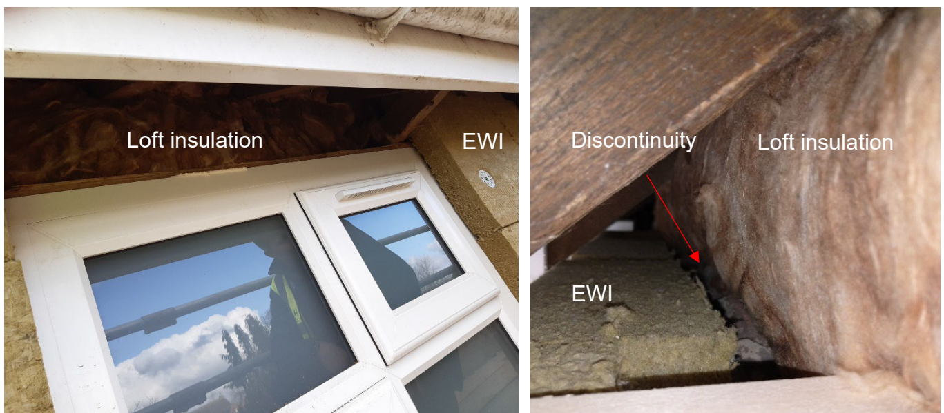
Figure 3-29 55AD EWI continuity with loft insulation at window heads junction (left), compared to EWI discontinuity at the external wall to ceiling junction (right)
