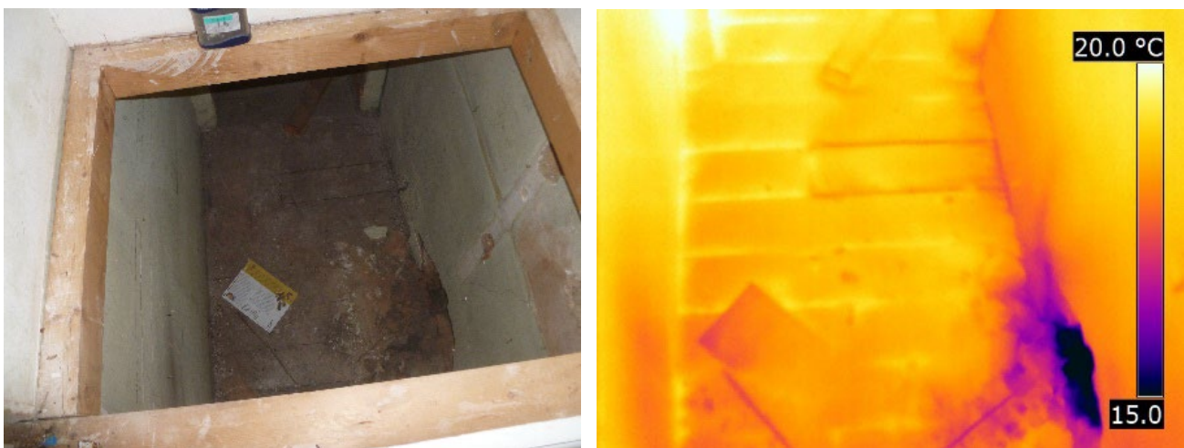
Figure 3-4 Air leakage via external wall opening in understairs area 57AD (hatch access only)
