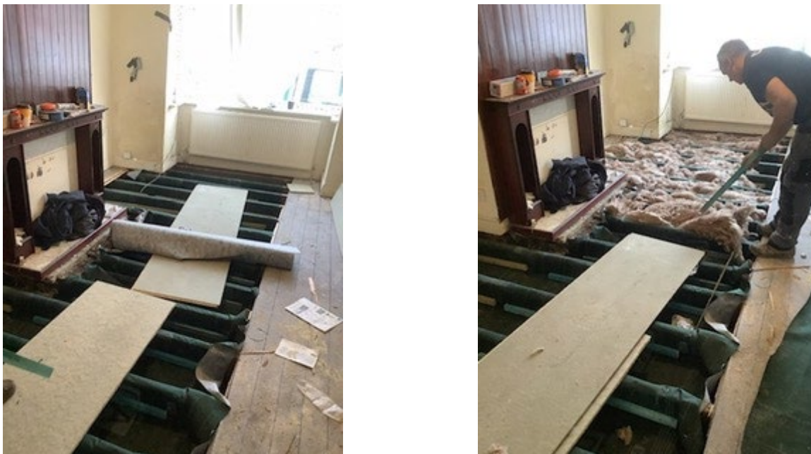
Figure 3-17 The airtight membrane was laid over and between floor joists in the living room (left hand side) and before the mineral wool insulation added (right hand side)
