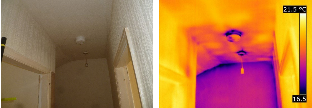
Figure 3-4 Air leakage around electrical penetrations in the landing
