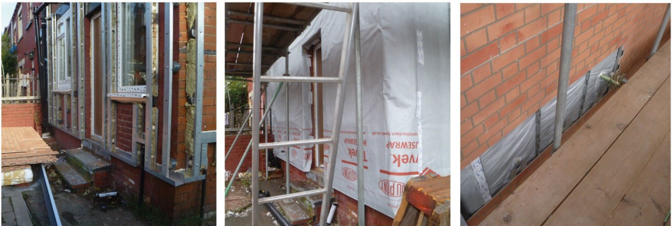
Figure 3-18 The EWI installation process. The steel section frame was put up (left hand side), then covered with a membrane and injected with insulation (middle). Finally, the pre-made rainscreen panels were added (right hand side).
