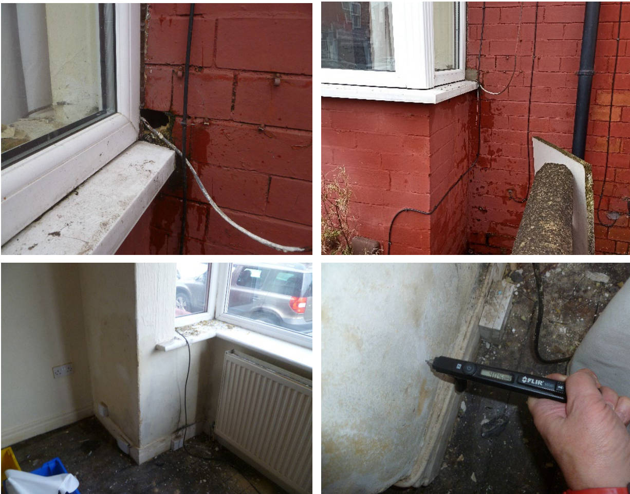
Figure 1-5 Evidence of damp in baseline case study
