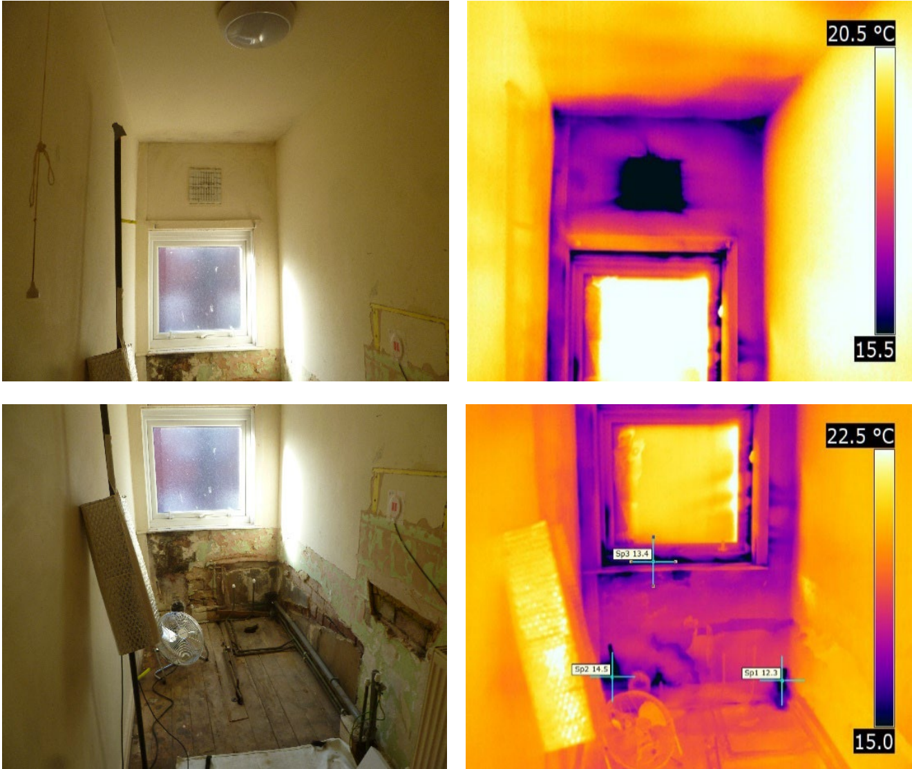
Figure 3-6 Air leakage around bathroom service penetrations at Stage 1 (01BA.B)
