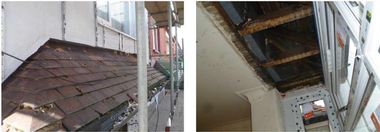
Figure 3-19 The bay window roof before rainscreen panels were added (left hand side) and internally, prior to insulation being installed (right hand side).
