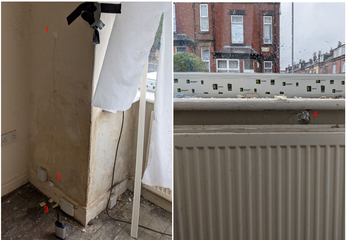
Figure 3-34 Position of thermocouple sensors in living room. Left: sensors on external wall. Right: sensor below window sill.
