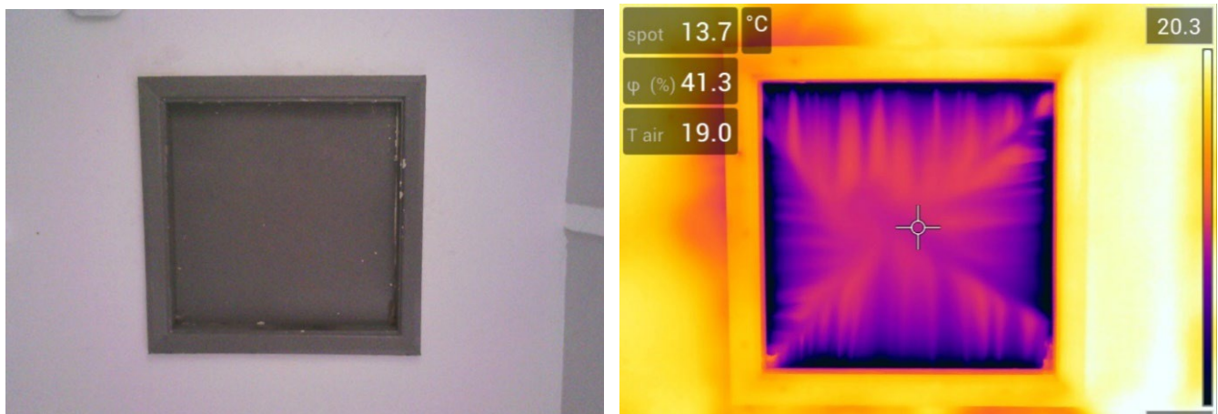
Figure 3-4 Infiltration at loft hatch edges during depressurisation pre-retrofit
