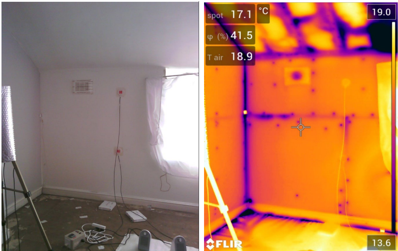
Figure 3-3 Infiltration at intermediate floor perimeter during depressurisation, pre-retrofit, also showing imperfectly installed sloping roof insulation, and existing thin internal wall insulation
