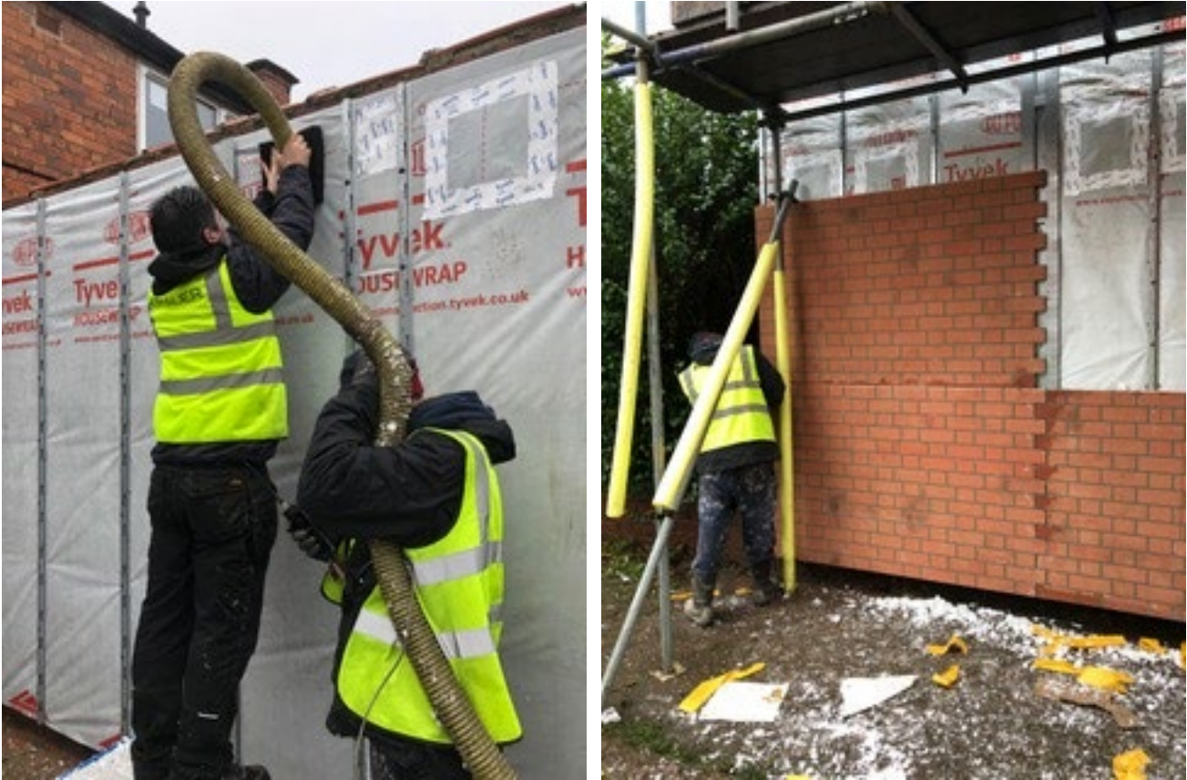
Figure 3-14 Blown mineral wool and brick effect panels EWI being fitted to the gable wall
