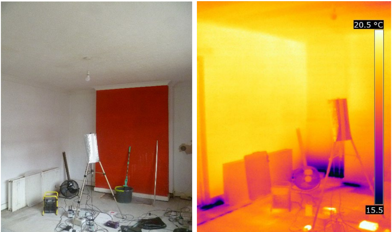
Figure 3-2 Infiltration at suspended floor perimeter during depressurisation post-retrofit
