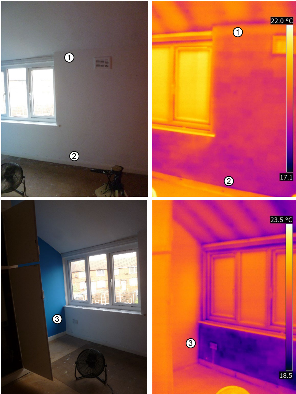
Figure 3-41 Photographs and IR images of rear wall showing position of surface temperature sensors. Top: 1 and 2. Bottom: 3
