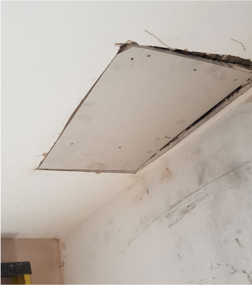
Figure 3-18 Ceiling removal to access loft to install insulation and replacement mid-installation (17BG.A.R.F.W.WH)
