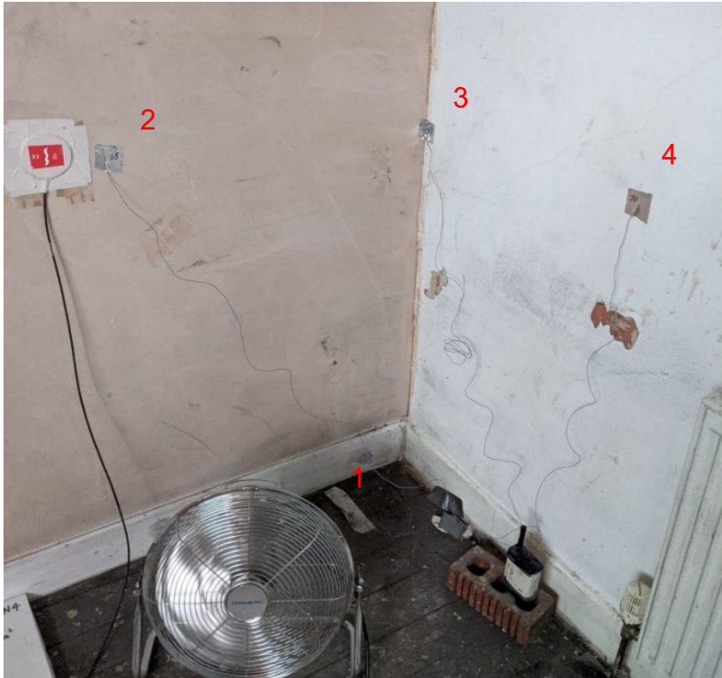
Figure 3-48 Room-in-roof thermocouple locations (17BG.W)
