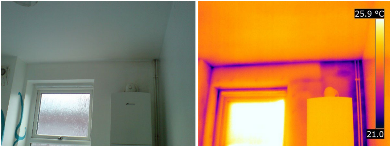
Figure 3-45 Existing TIWI installed to the left of the boiler (warmer), uninsulated wall above and to the right of the boiler (colder)
