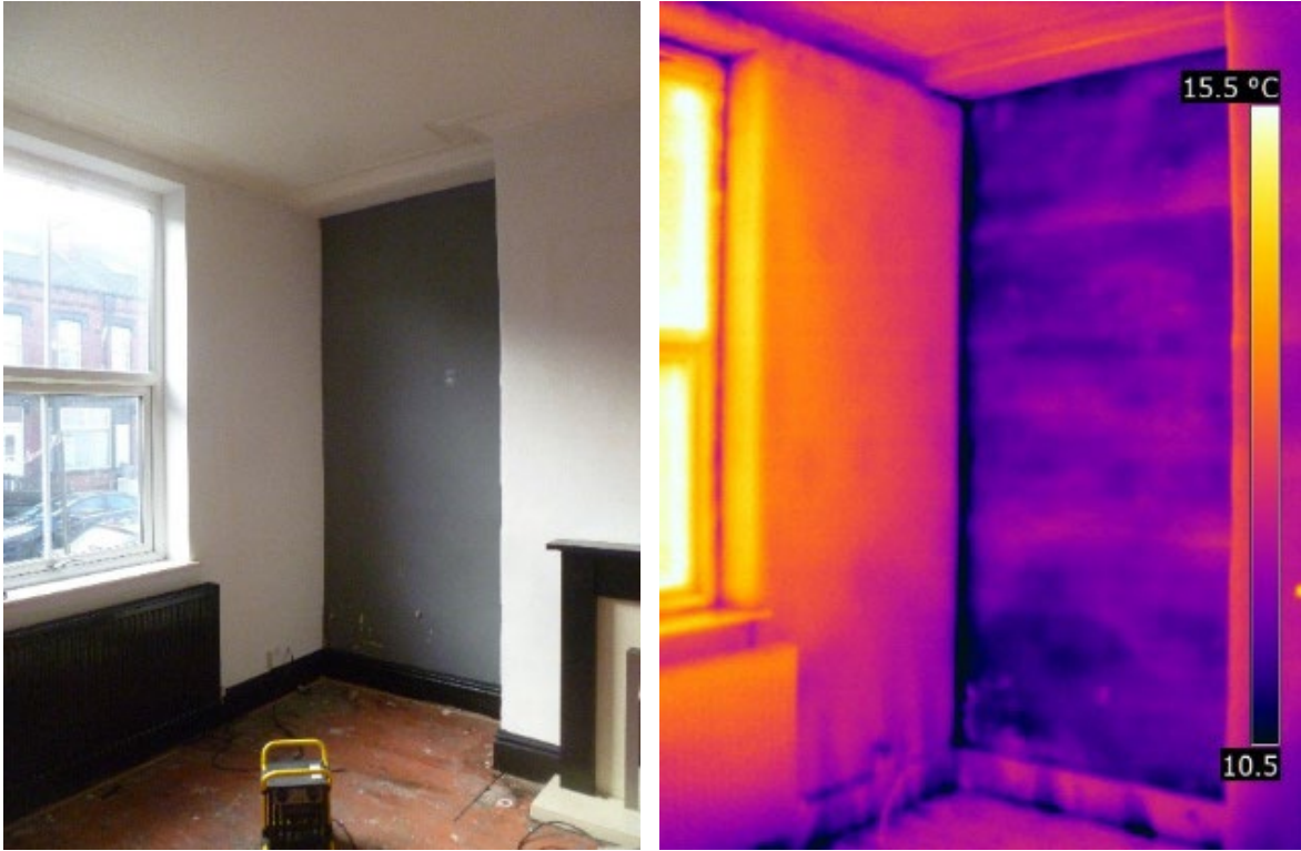
Figure 3-1 Base case infiltration through the suspended timber ground floor at wall junction and behind the existing IWI during depressurisation
