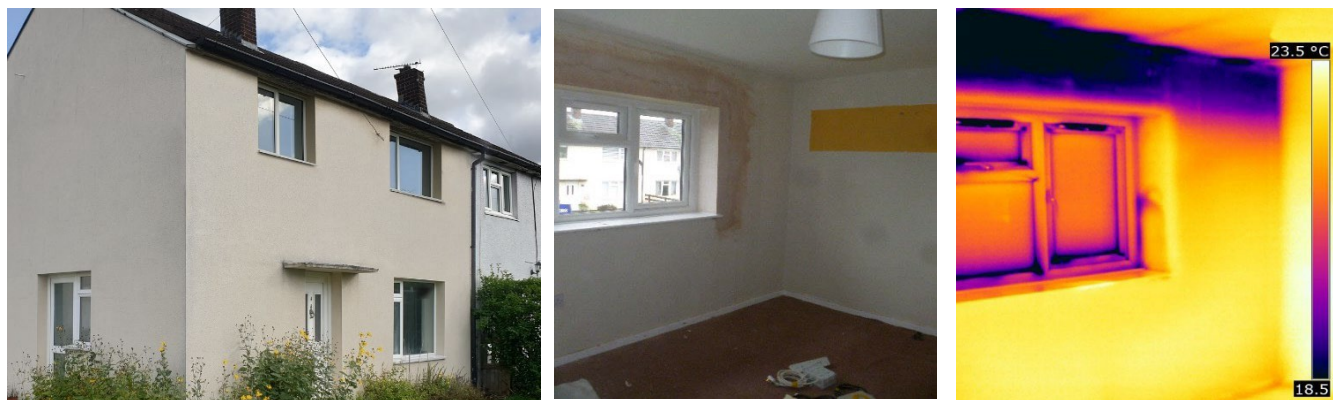
Figure 1-22 Thermal bridge where EWI does not extend to the eaves
