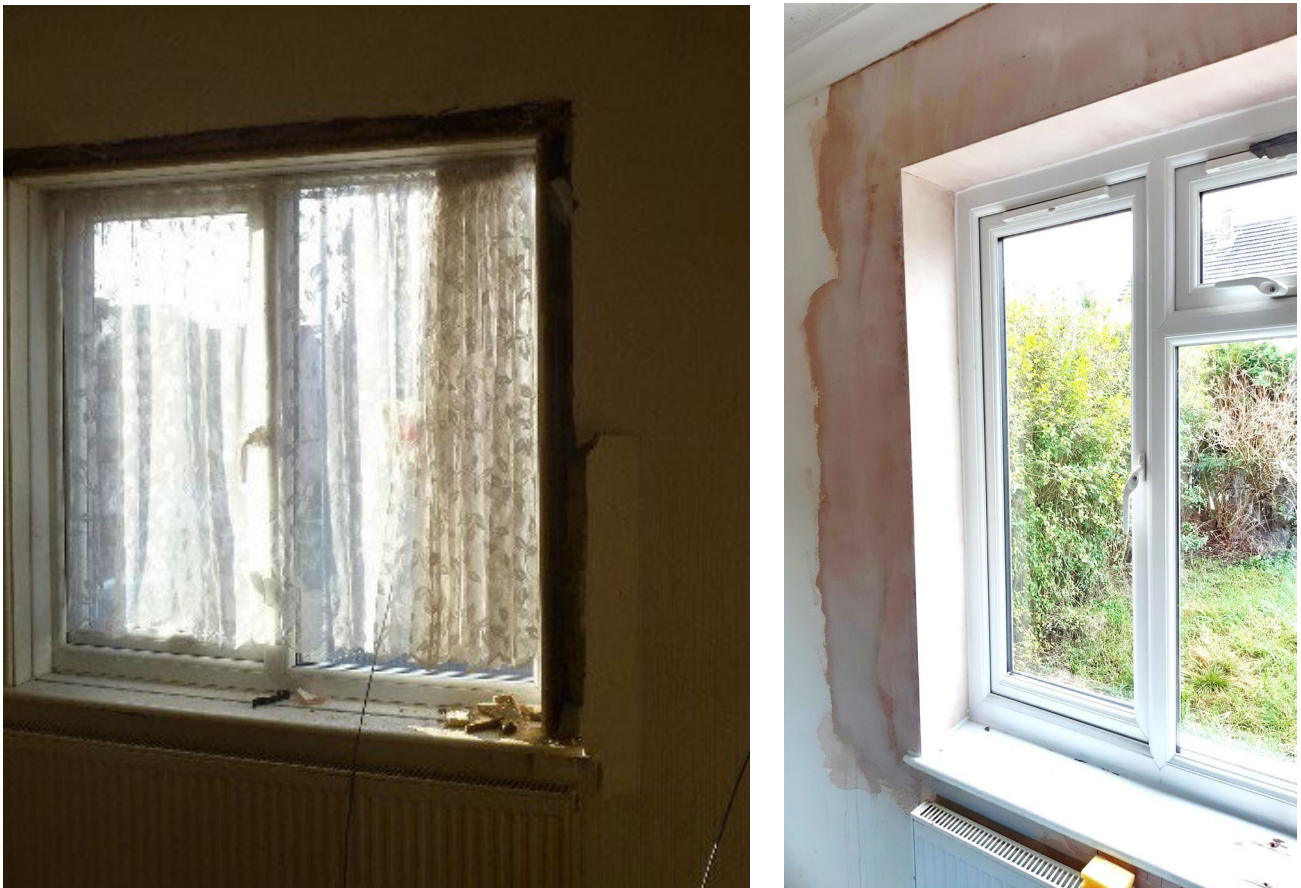
Figure 1-15 Damage caused during window installation
