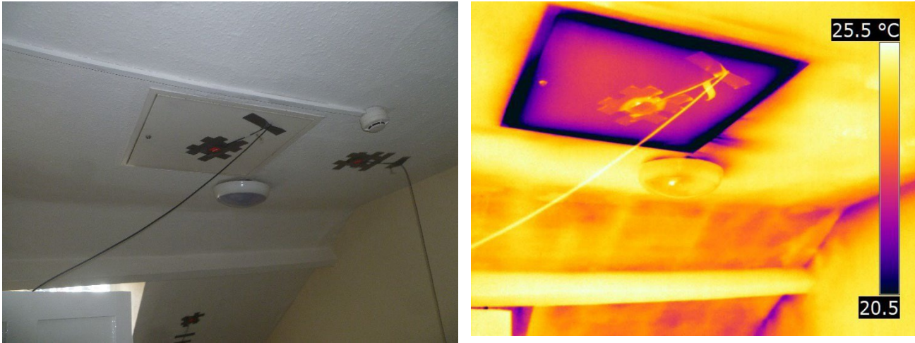
Figure 1-11 Example of unsealed and uninsulated loft hatch
