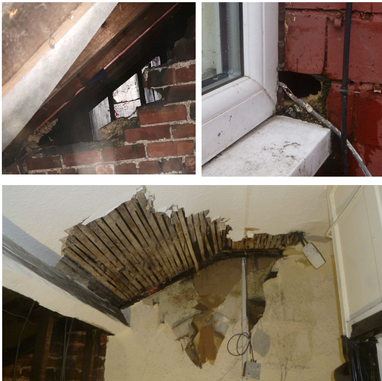
Figure 4-2 Examples of repair issues in DEEP case study homes (Top left; incomplete party wall, Top right; damage to masonry, Bottom; leak in roof)
