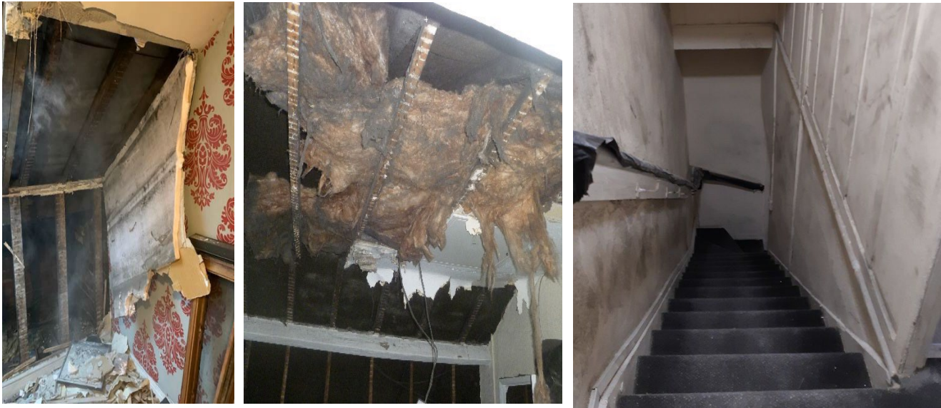
Figure 1-12 Disruption and excessive soot caused during room-in-roof retrofit
