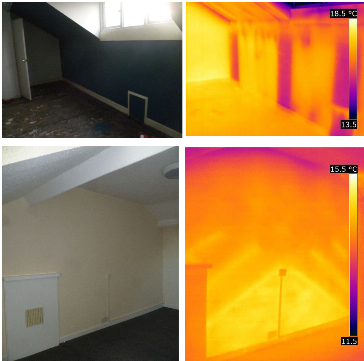
Figure 5-4 Heterogenous heat losses through fabric caused by variations in construction (top, missing insulation in a stud wall, bottom, varying construction in party wall)
