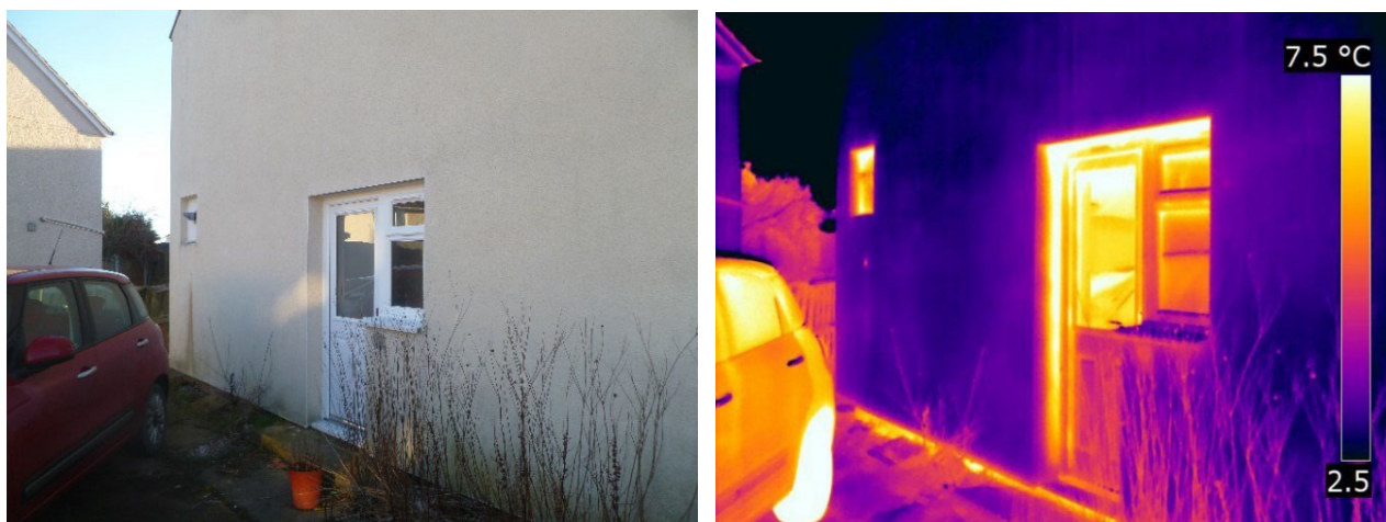
Figure 1-21 Thermal bridge around boiler flue and below DPC caused by EWI discontinuities
