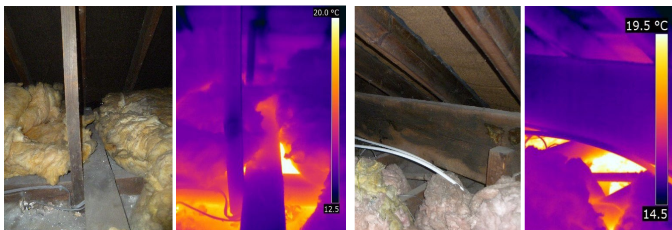
Figure 1-10 Disturbed loft insulation in case study home causing thermal bridging (left: insulation moved to install wiring, right: Purlin obstructing access to insulate)
