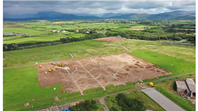
An aerial view of the herringbone drainage, installed during the STIM early works
