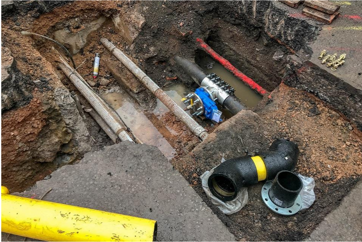
Figure 1: Roads carry utility pipes providing essential services, and are excavated to maintain and repair this infrastructure. Source: © Crown copyright.
