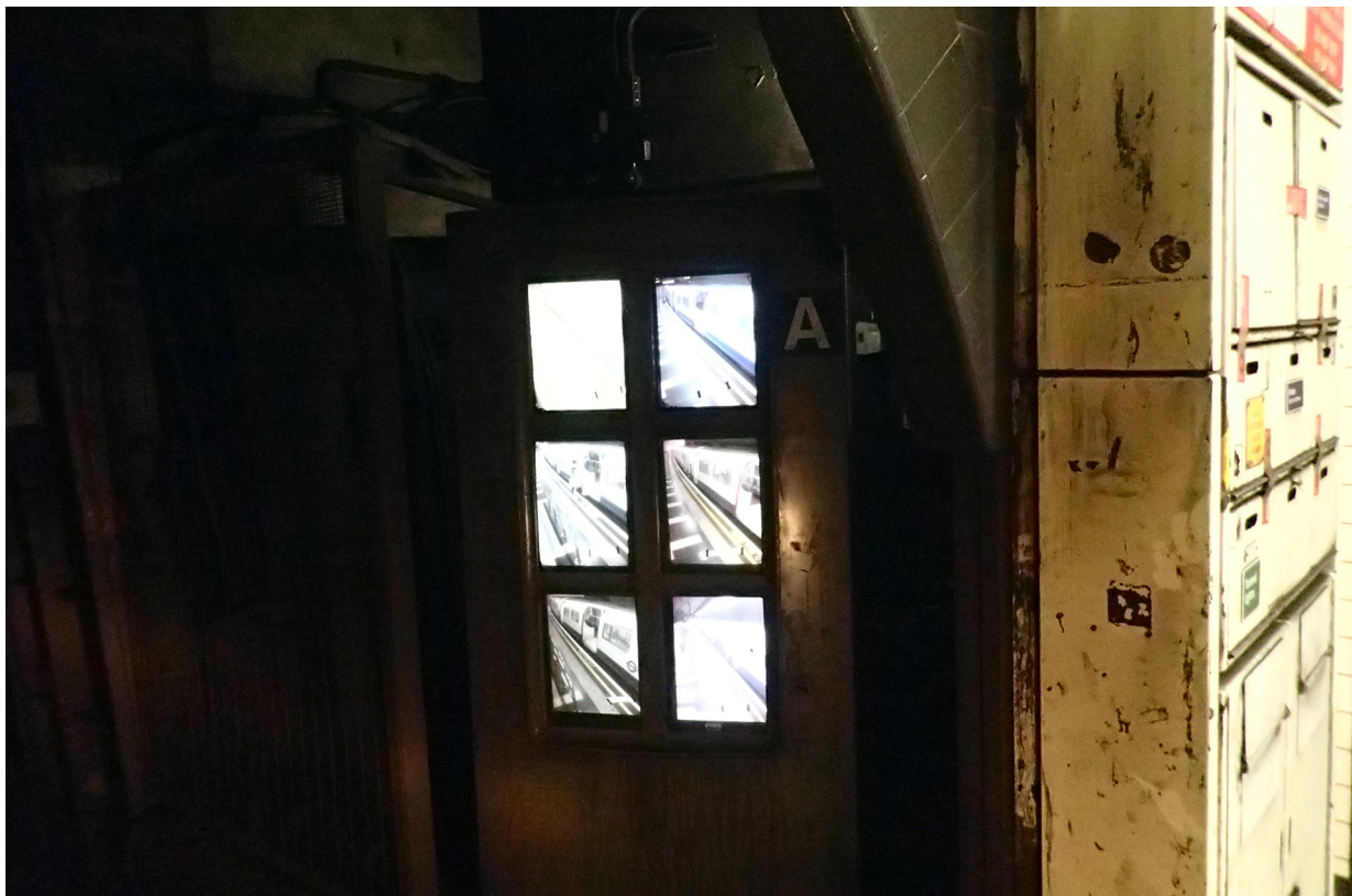
Figure 5: OPO monitors provided inside the tunnel at Waterloo Bakerloo line platform 3
