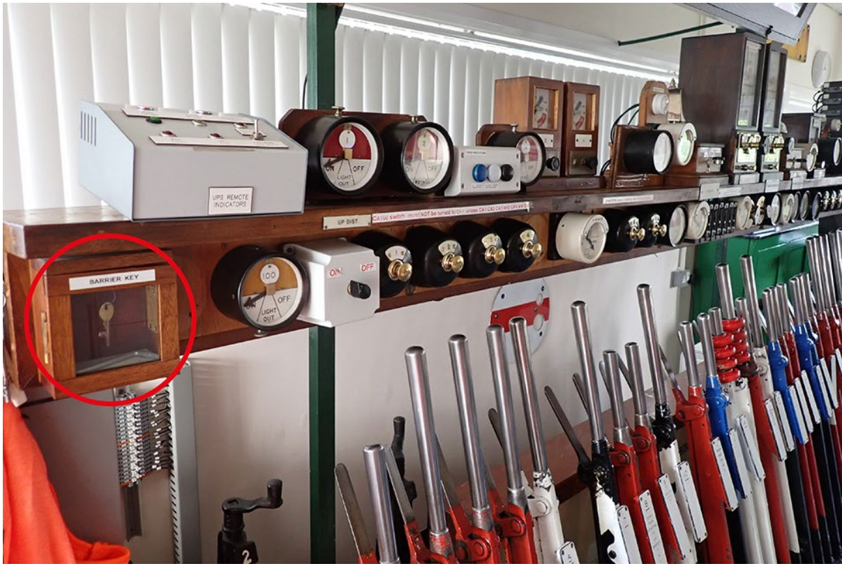
Craven Arms signal box block shelf, showing the key used to access the LCU.
