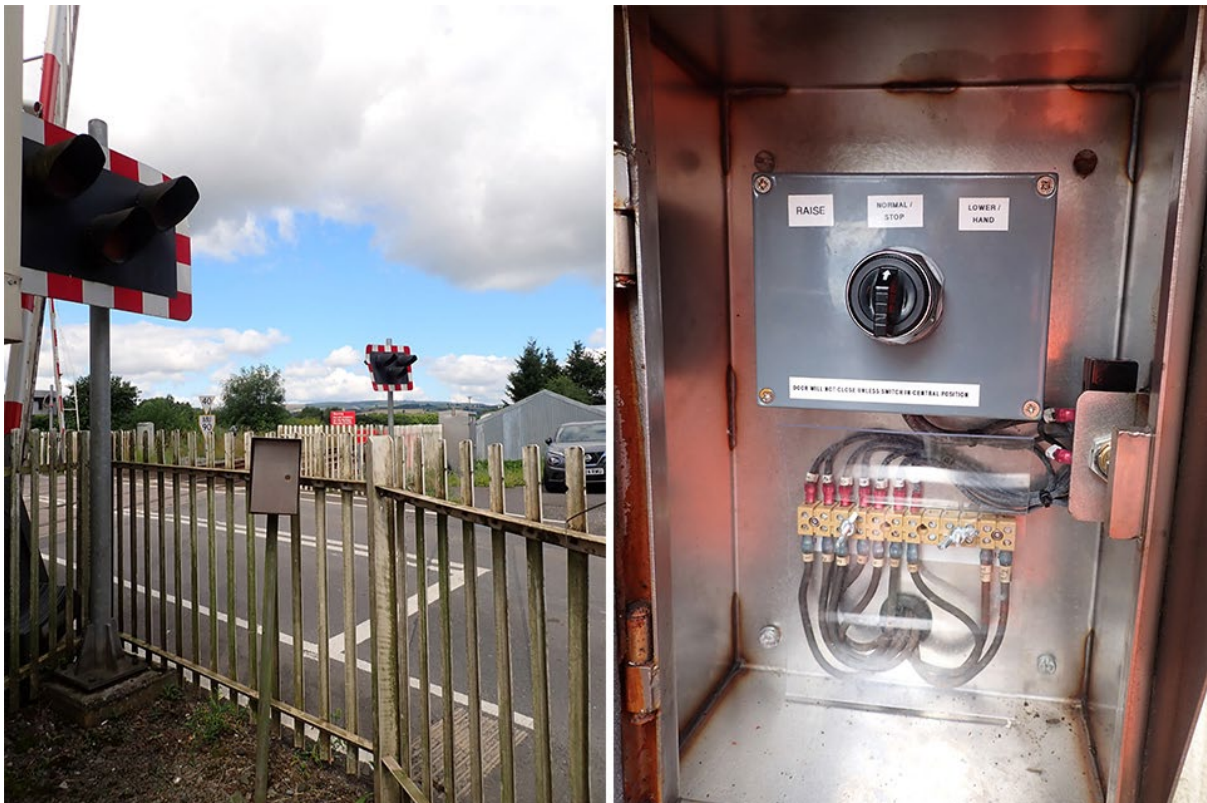
LCU located outside of the signal box (left). LCU's internal switch (right).
