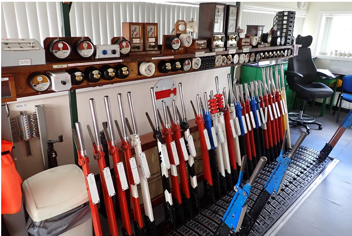
Craven Arms signal box lever frame. For illustrative purposes the red levers are 'in the frame' in their normal positions. If they were to be pulled 'out of the frame' to their reverse positions they would be on the right-hand side of the image, similar to the blue levers.
