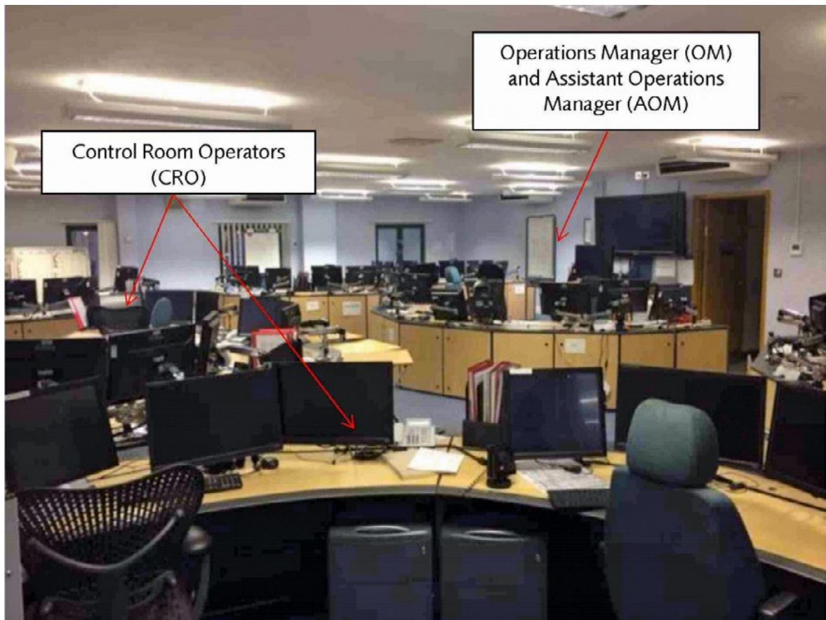
Figure 7.2 The Stratford Control Room
