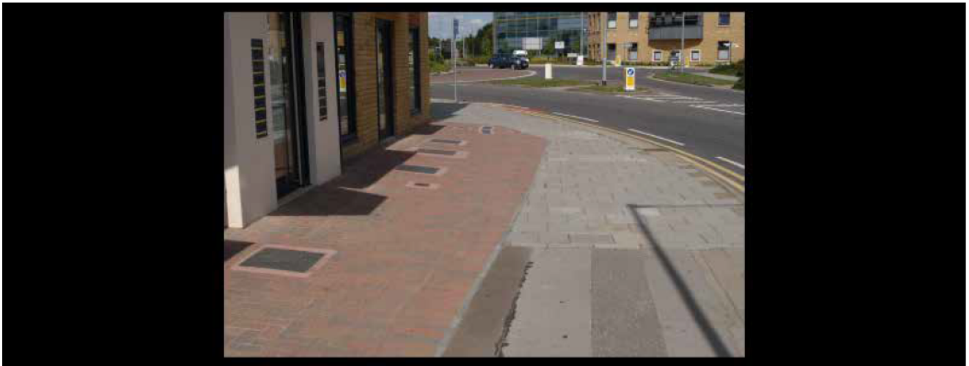
What not to do: plot demarcation ignoring the existing footway creates a disjointed public realm
