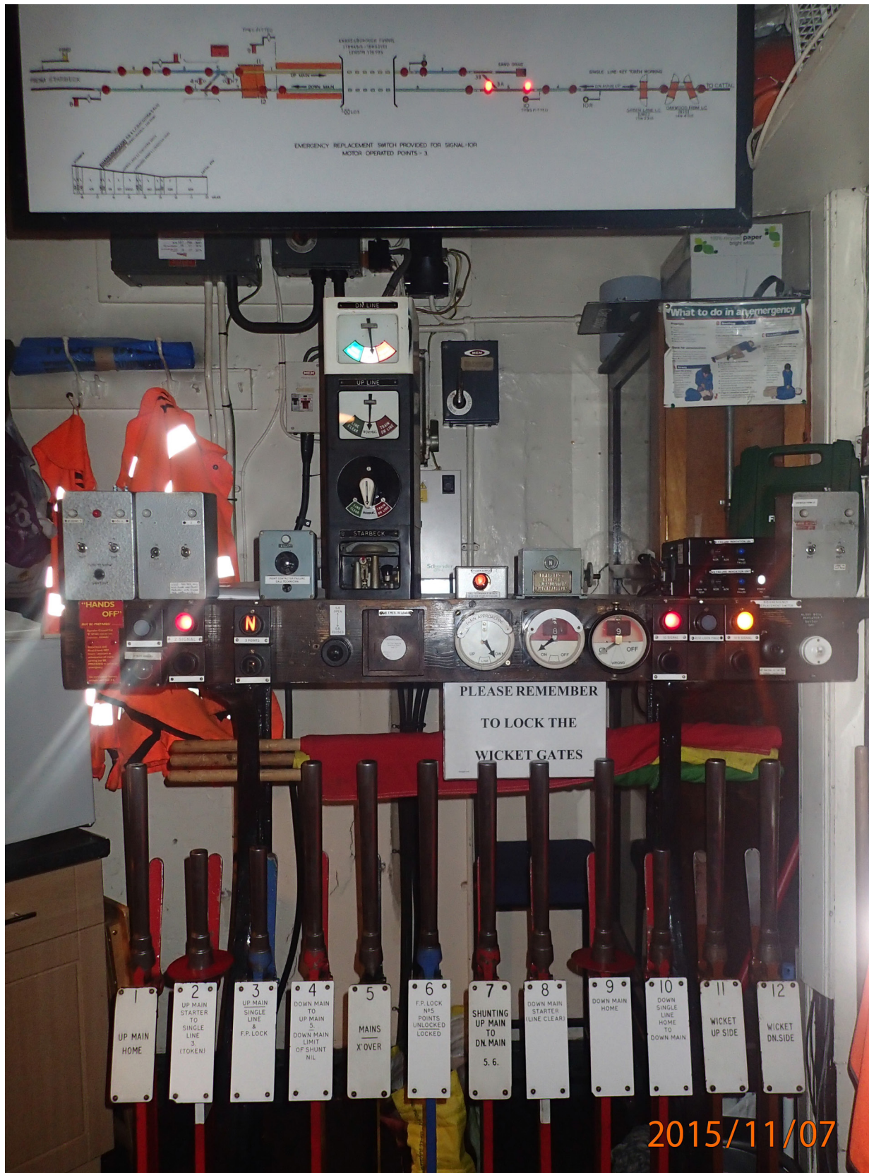
Figure 5: Knaresborough signal box lever frame
