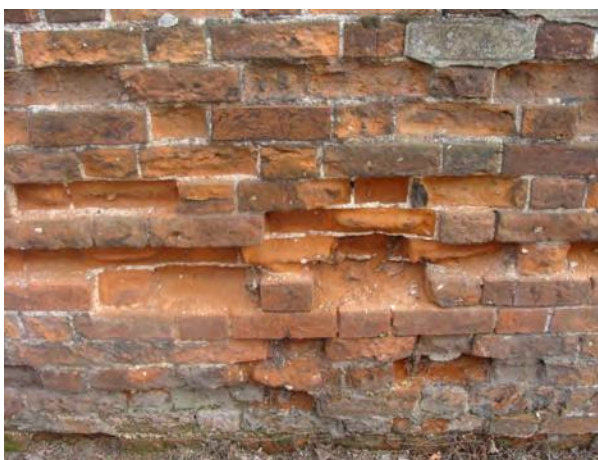
Picture 1.18 Garden wall to The Grange, Church Street, in urgent need of repair
