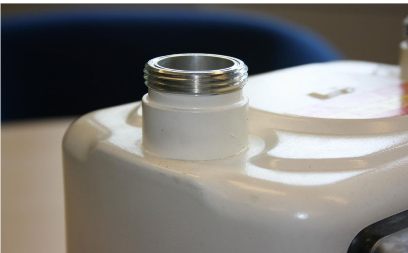
Gas meter – No rust over meter boss
