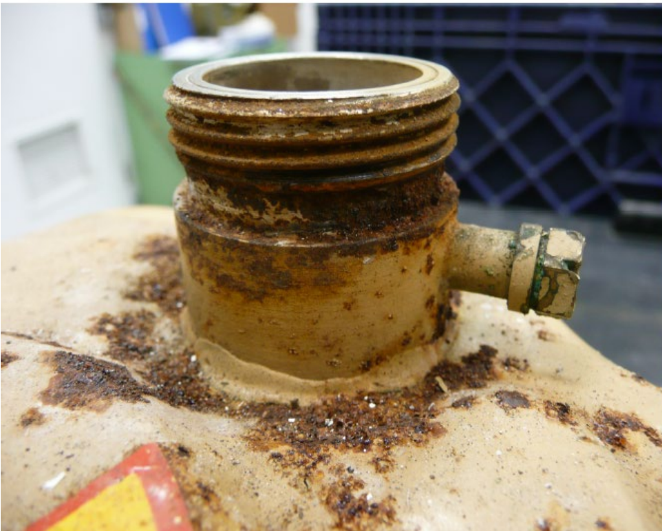
Gas meter – Medium level of rust on boss
