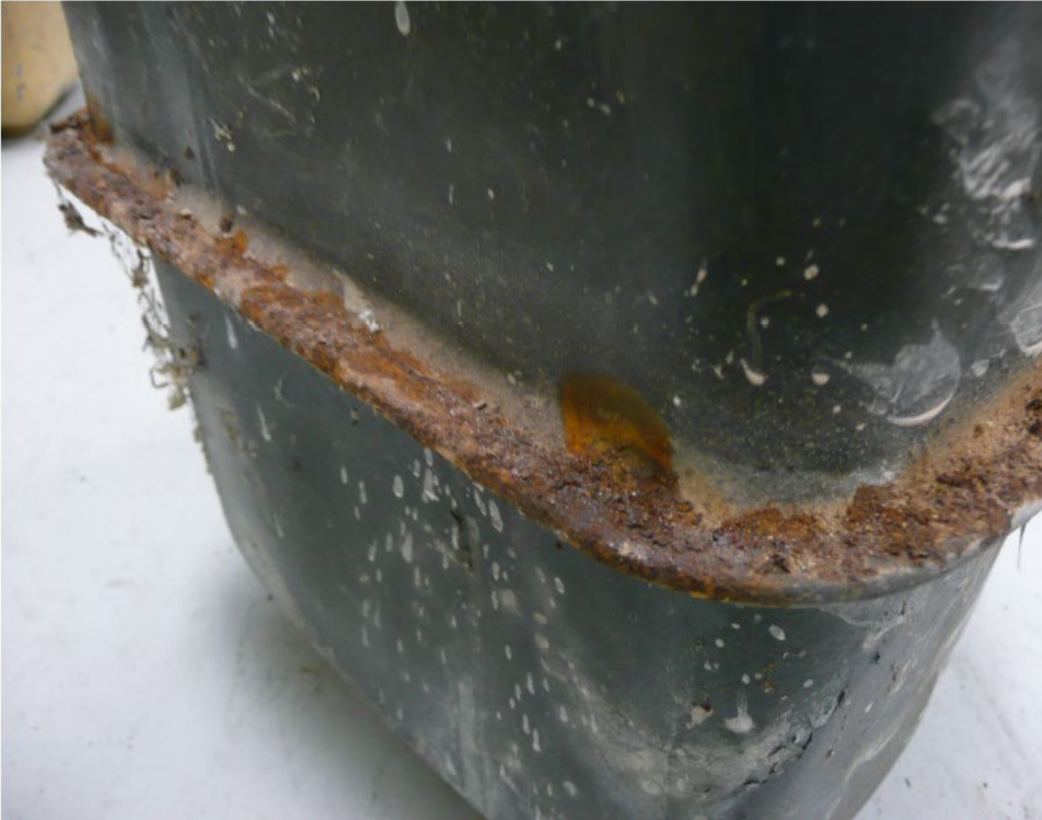
Gas meter – Medium level of rust on band
