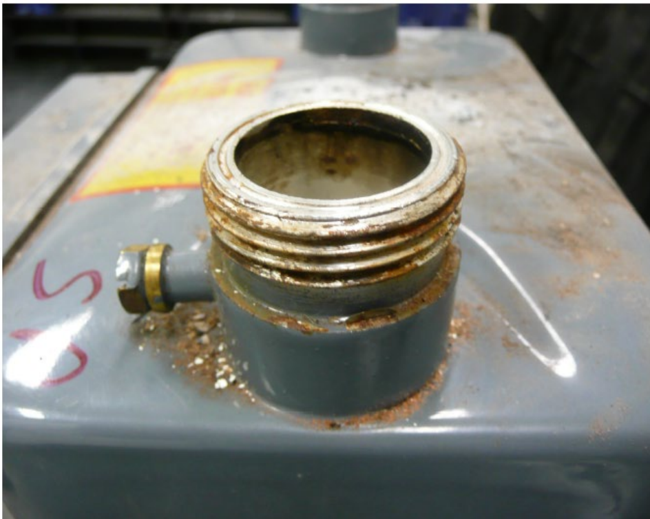
Gas meter – Low level of rust on boss
