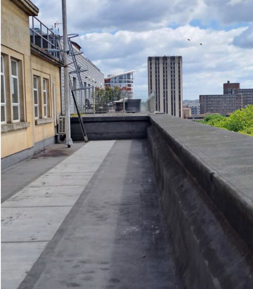
Photograph 8: Maintenance ladder to roof (access maintained via gate in new partition screen)
