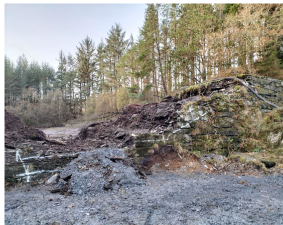
Figure C3.2: View of downstream face of dam structure following completion of excavation (source: Dr Andrew Hughes, Dams and Reservoirs Ltd)
