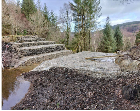
Figure C3.6: View of dam structure from upstream following completion of works (source: Dr Andrew Hughes, Dams and Reservoirs Ltd)
