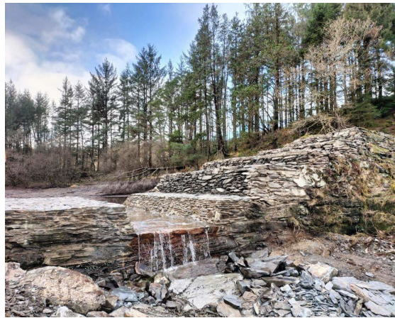
Figure C3.4: View of downstream face of dam structure following completion of spillway and sidewall construction (source: Dr Andrew Hughes, Dams and Reservoirs Ltd)
