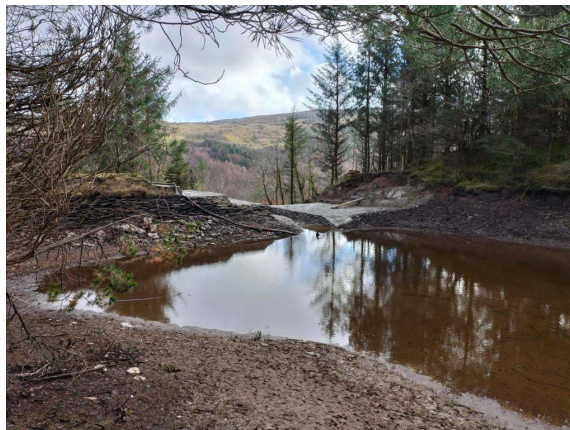
Figure C3.5: View of dam structure from upstream following completion of works (source: Dr Andrew Hughes, Dams and Reservoirs Ltd)
