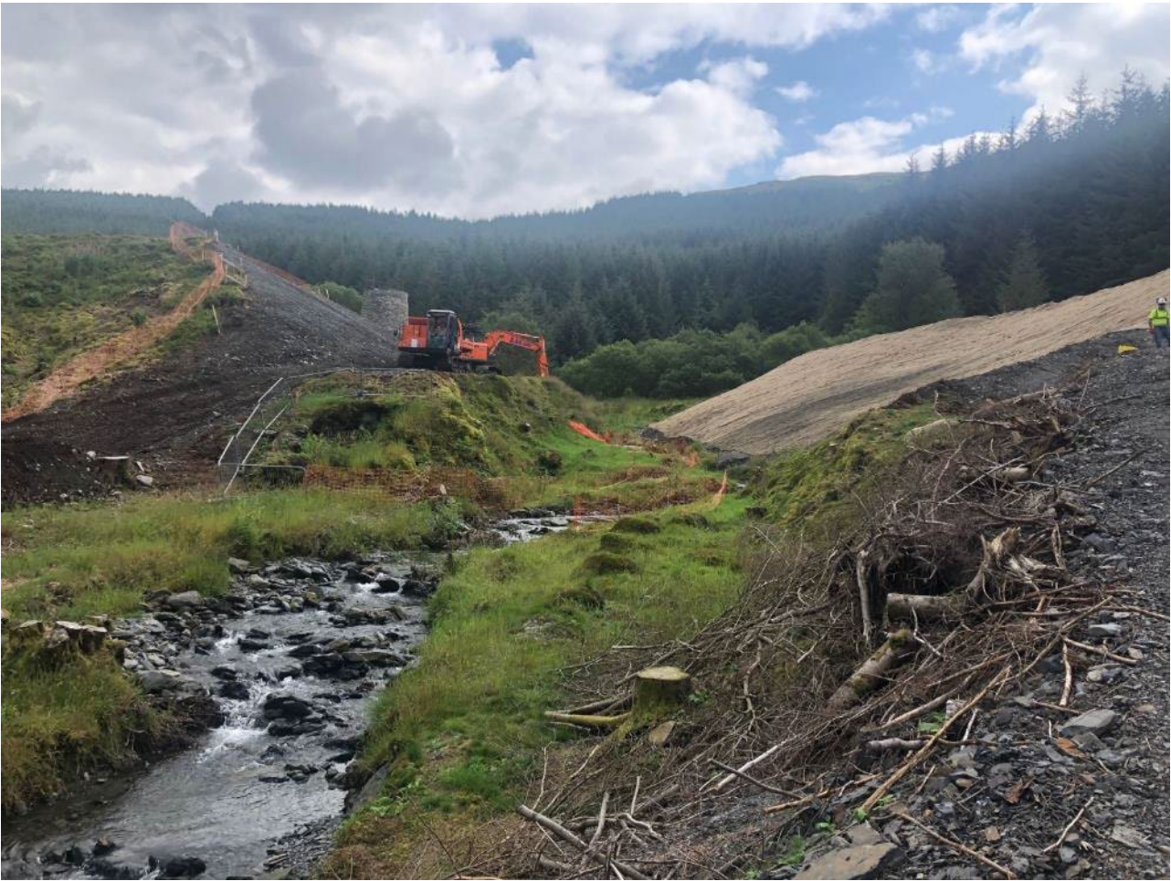
Photograph 4: Excavating through an embankment dam (source: Dr Andrew Hughes, Dams and Reservoirs Ltd)
