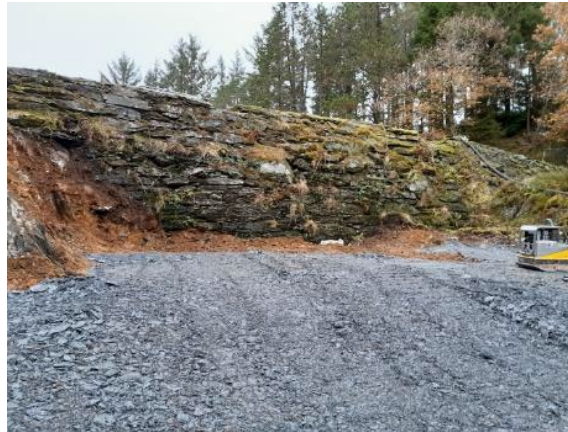
Figure C3.1: View of downstream face of dam structure following installation of access track at downstream toe (source: Dr Andrew Hughes, Dams and Reservoirs Ltd)
