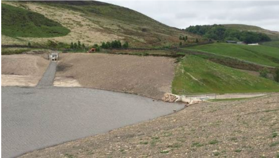
Figure C4.3: An image of the notch and works carried out on Sunnyhurst Hey Reservoir (source: Dr Andrew Hughes, Dams and Reservoirs Ltd)
