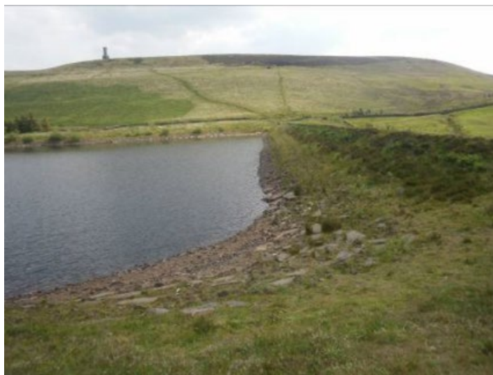
Figure C4.4: The original southern embankment where the work was carried out on Sunnyhurst Hey Reservoir (source: Dr Andrew Hughes, Dams and Reservoirs Ltd)
