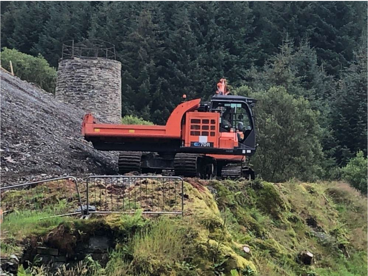
Photograph 5: Tracked dump truck with rotating body (source: Dr Andrew Hughes, Dams and Reservoirs Ltd)
