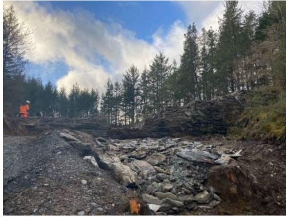
Figure C3.3: View of downstream face of dam structure following completion of spillway and sidewall construction (source: Dr Andrew Hughes, Dams and Reservoirs Ltd)
