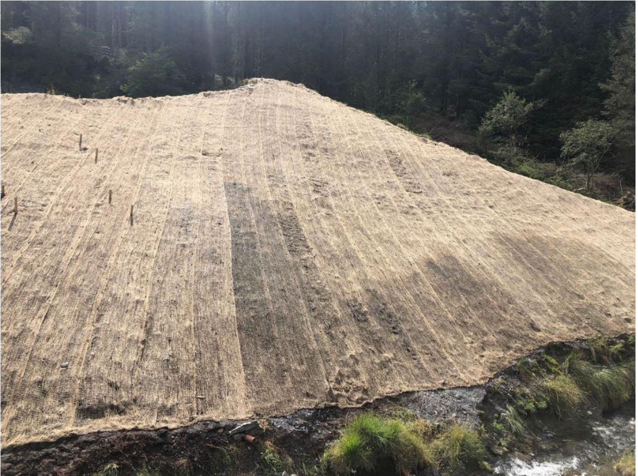
Photograph 7: View of cut slope protected with erosion protection matting (source: Dr Andrew Hughes, Dams and Reservoirs Ltd)
