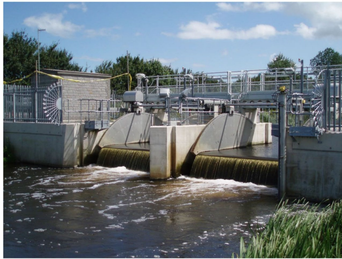
Figure 8: Greylake sluice on King's Sedgemoor Main Drain in Somerset which comprises 2 bottom-hinged tilting weirs (source: Andy Don)
