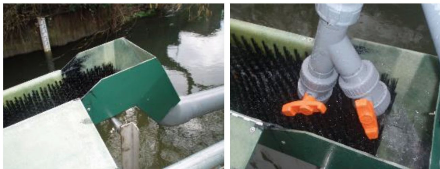
Figure 20: Effective flow splitter arrangement in use in Somerset (source: Andy Don)
