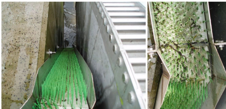
Figure 9: Pumped up-an-over eel pass at Greylake Sluice in Somerset (source: Andy Don)
