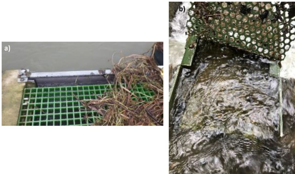
Figure 25: a) Glass reinforced plastic (GRP) cover at Tallington fish pass in Lincolnshire b) Damaged cover on a box section pass at Church Rd in Hampshire (source: a) Hugh Bunker/James Hooker, b) Kerry Sims)
