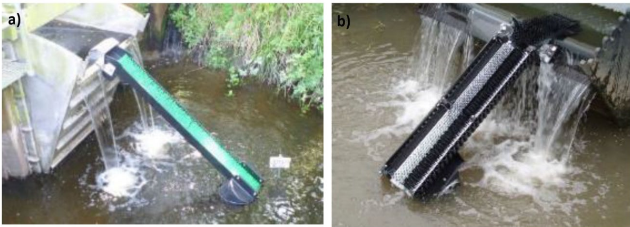
Figure 19: Two images of self-adjusting passes at sluice gates (source: a) Paula Rosewarne and b) Environment Agency, 2011a)
