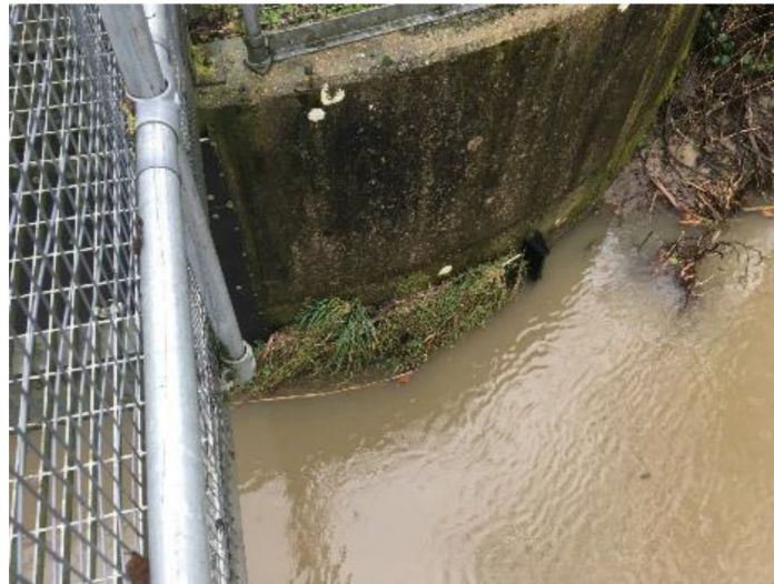
Figure 24: Debris accumulation and plant growth on the vertical bristle board section of an eel pass at Partney in Lincolnshire (source: Lesley Shuttleworth)
