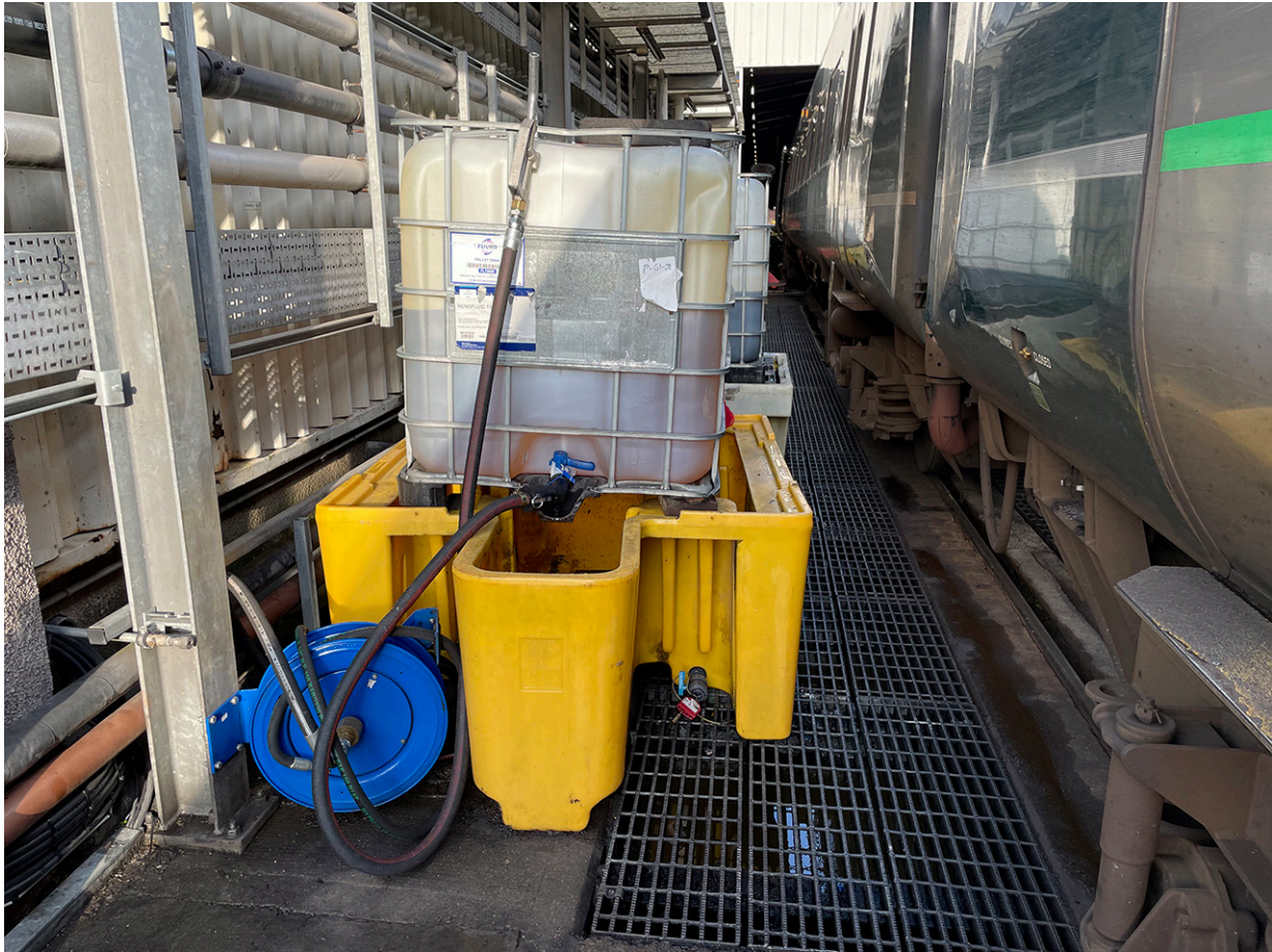
Figure 9: The intermediate bulk containers.
