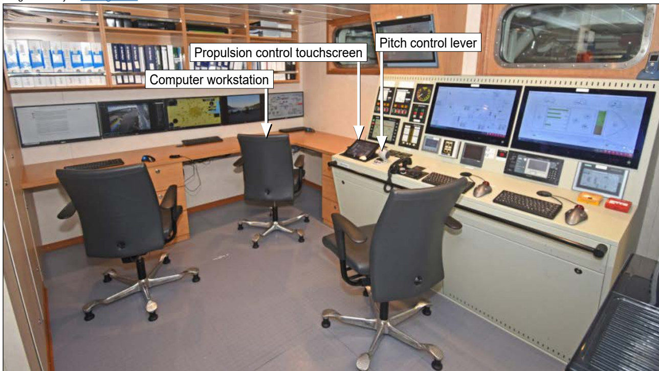
Figure 3: The engine control room
