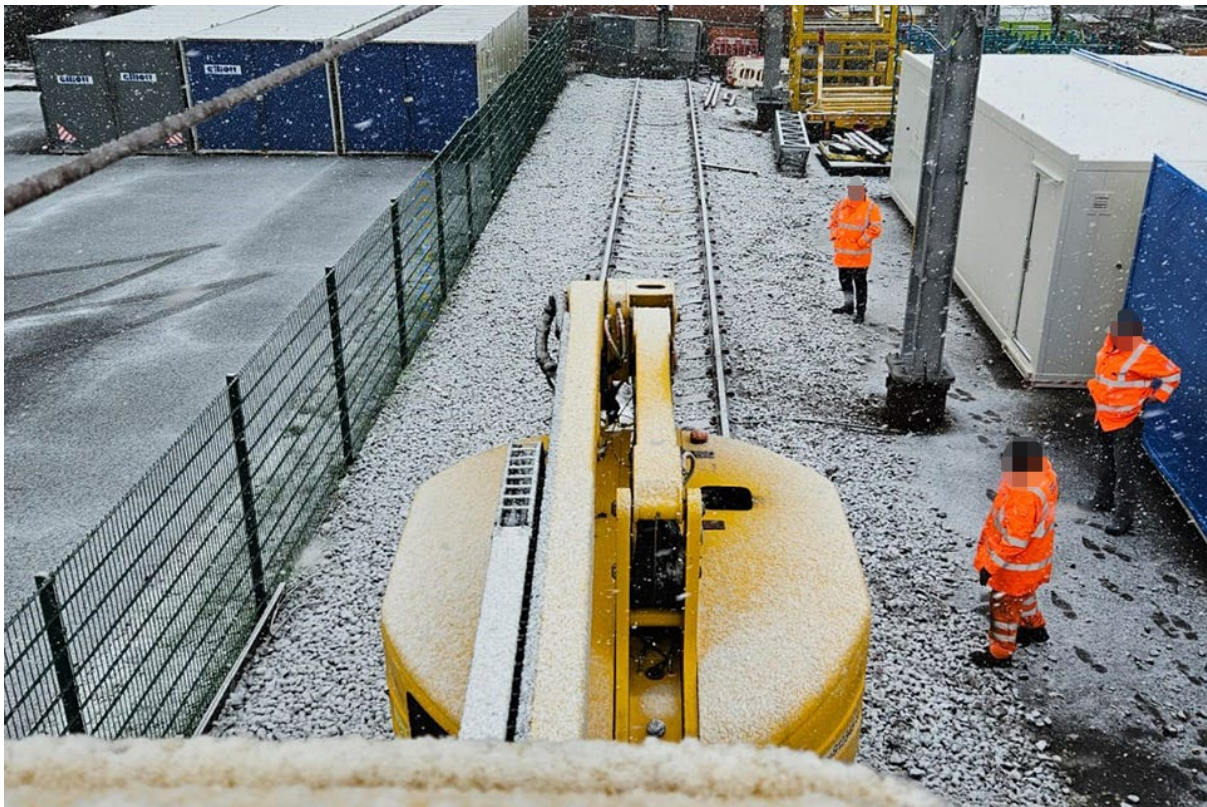
View from the raised operator's basket showing the restricted view of the track immediately ahead of the machine. (Courtesy of SPL Powerlines UK Ltd.)
