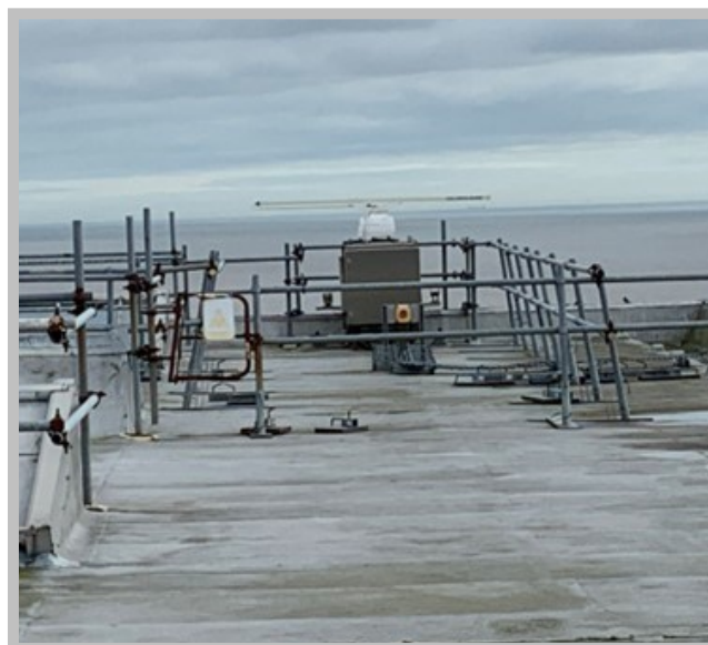
Figure 8: CEFAS Radar on Reactor Building Roof
