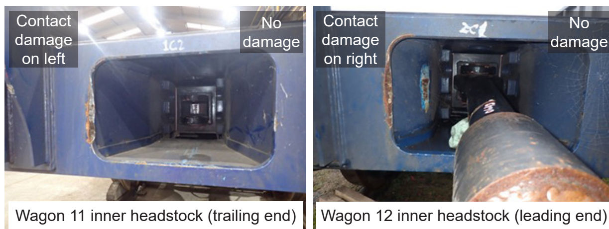
Figure 14: Witness marks on the headstock pockets on wagon 11 and wagon 12 after recovery (rigid drawbar is shown disconnected from wagon 11, and after a weld repair had been done).
