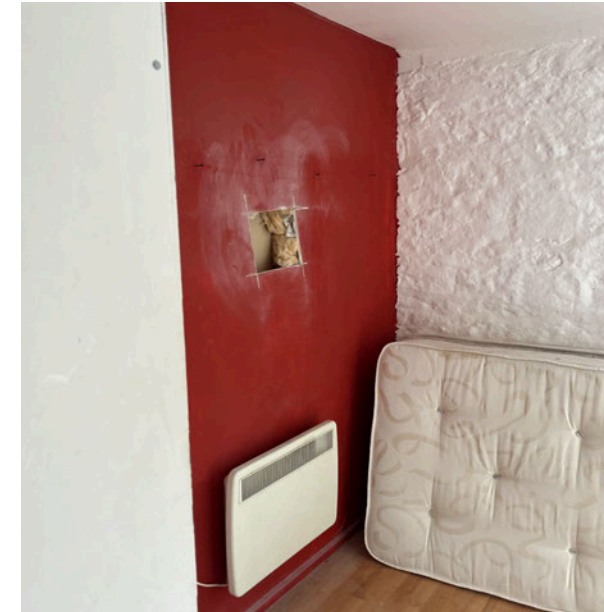
Low quality stud walls
