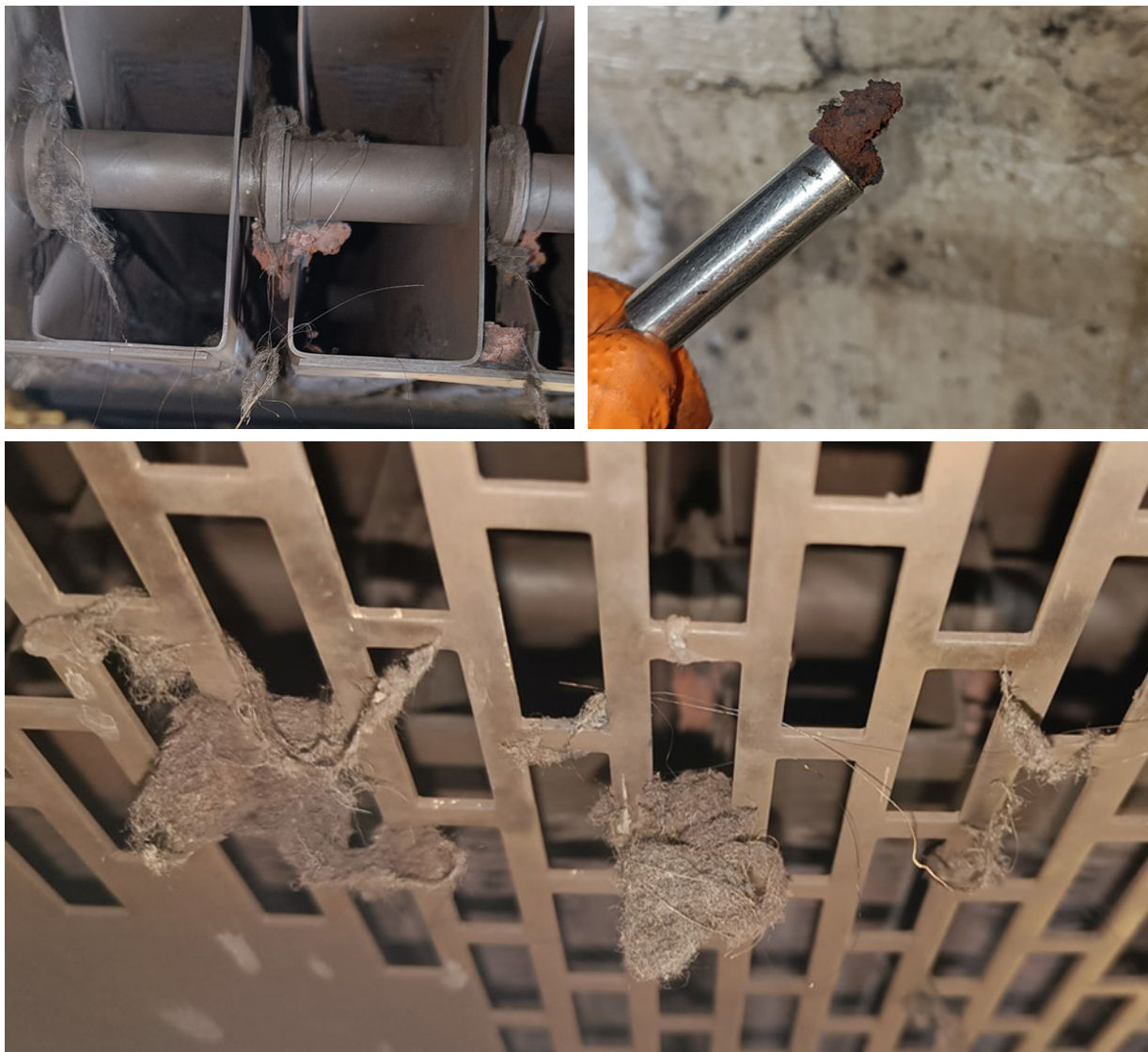
Figure 15: Remaining material found on brake resistor of car 4 of train 065 following the incident. Top left-hand image shows red magnetic clay on inlet to the resistor, bottom image shows organic material on the resistor grid and top right-hand side image shows red magnetic clay material (before material testing). Courtesy of LUL.
