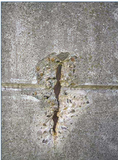
Figure 5.3 Spalling of concrete over corroding reinforced bar, where cover is reduced by groove feature (courtesy CH2M Hill, with permission from the Environment Agency)
