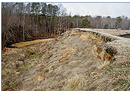
Figure 5.5 Slumping of earth embankment
