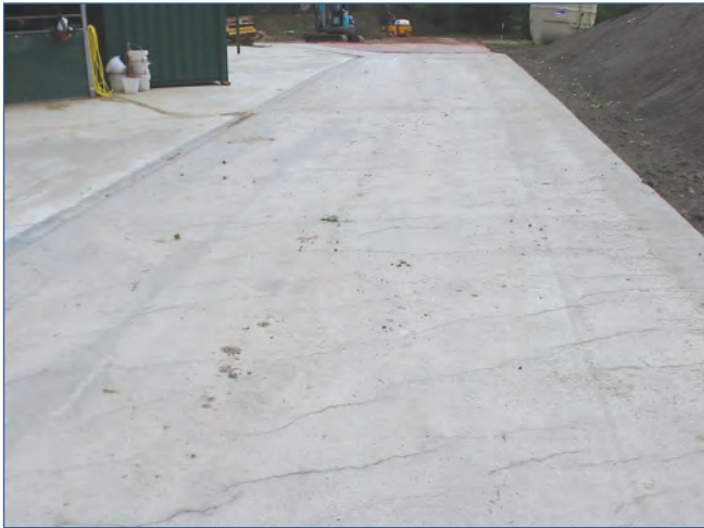
Figure 7.6 Plastic shrinkage cracks (courtesy Concrete Society)
