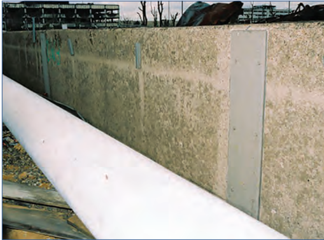
Figure 5.11 A plated joint (courtesy CH2M Hill, with permission from the Environment Agency)
