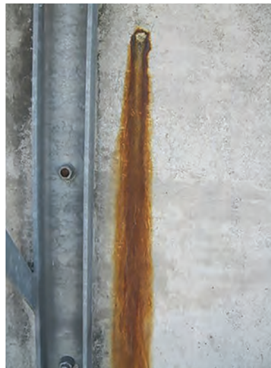
Figure 5.4 Rust staining that may indicate corroding reinforcement (or a metal fixing) (courtesy CH2M Hill, with permission from the Environment Agency)
