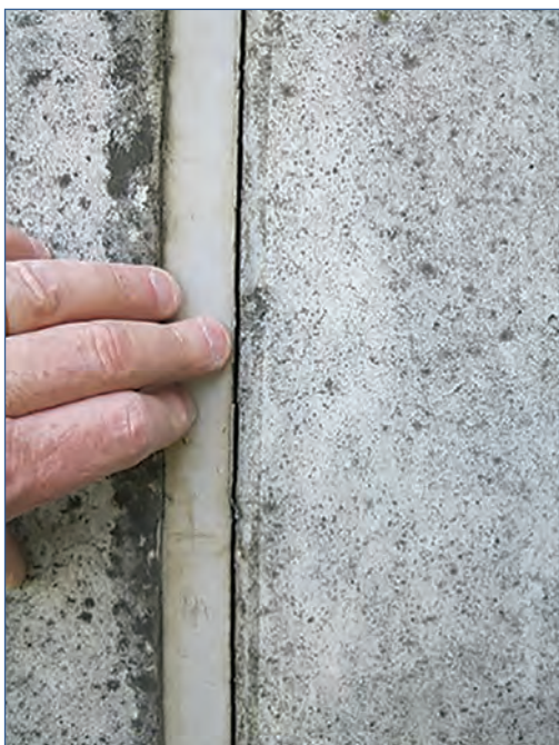
Figure 5.15 Over time, sealants will detach from the sides of joints and must be regularly inspected and replaced (courtesy CH2M Hill, with permission from the Environment Agency)
