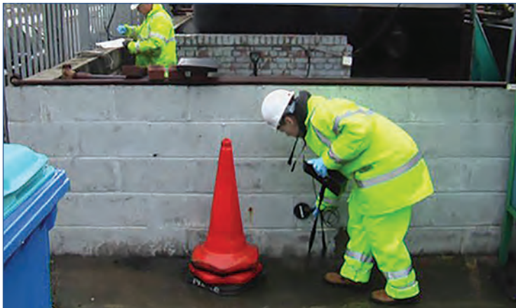
Figure 5.9 A cover meter survey (courtesy CH2M Hill, with permission from the Environment Agency)
