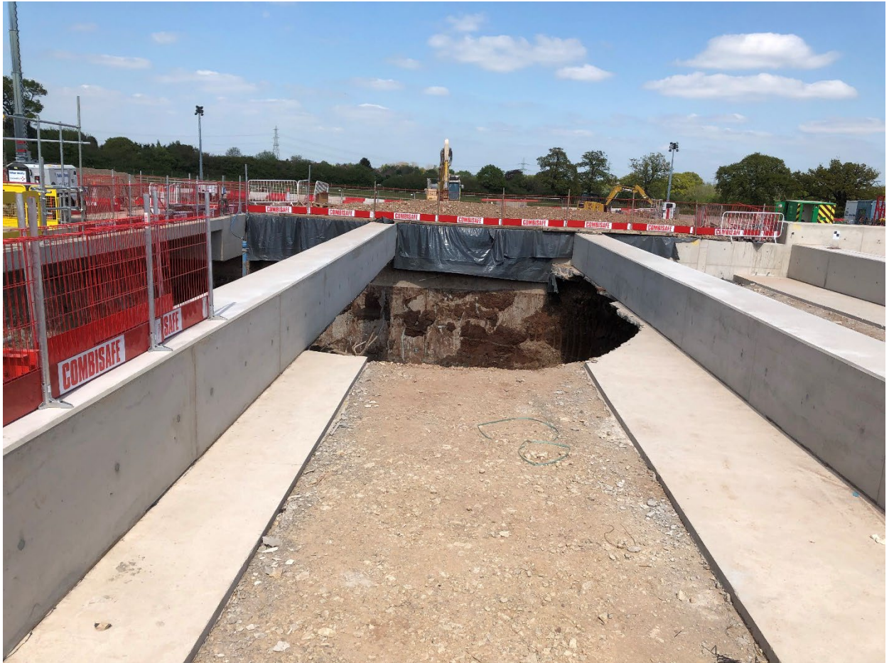
View looking northwards across the cutting, showing in-situ concrete props running between the northern and southern retaining walls and the partial excavation of the ground between a pair props
