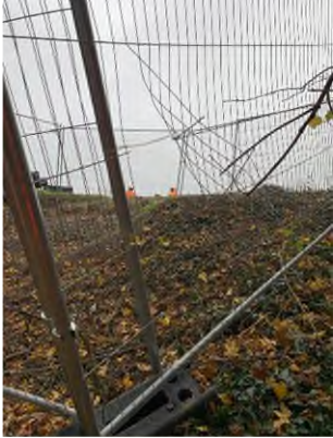
Damage to Heras fence
