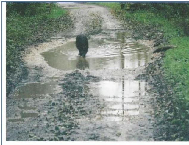
Condition of Lower Track prior to Residents investing over £120k in new surface
