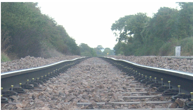
An example of poor track geometry which resulted in derailment of a freight train.
