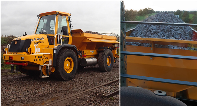
Ballast distributor RRV, and the view from the cab when running in reverse.
