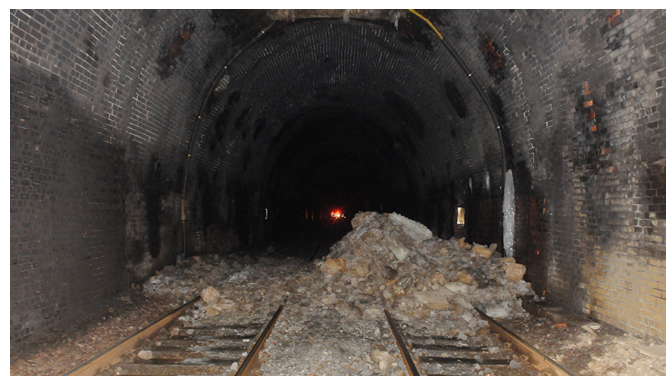
Ice found below a ventilation shaft after the derailment at Summit tunnel (courtesy of British Transport Police).
