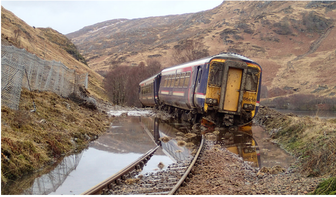
Derailed train following landslip at Loch Eilt.
