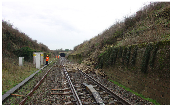
Collapsed wall following landslip at Kemble.
