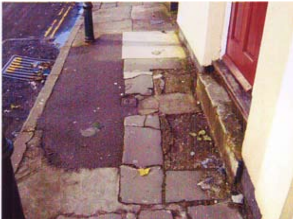
Figure 137: A dangerous, unsightly mix of pennant, tarmac and concrete on Princess Victoria Street
