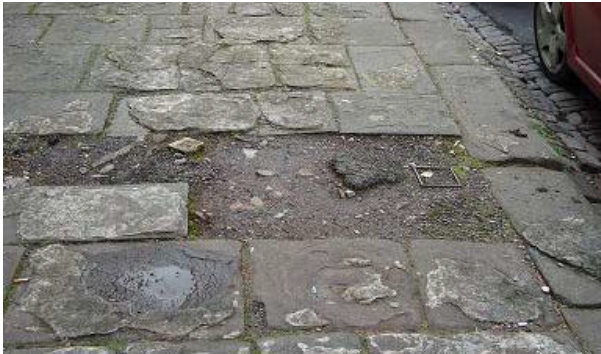
Figure 136: This pennant paving on a Grade II terrace is sorely neglected
