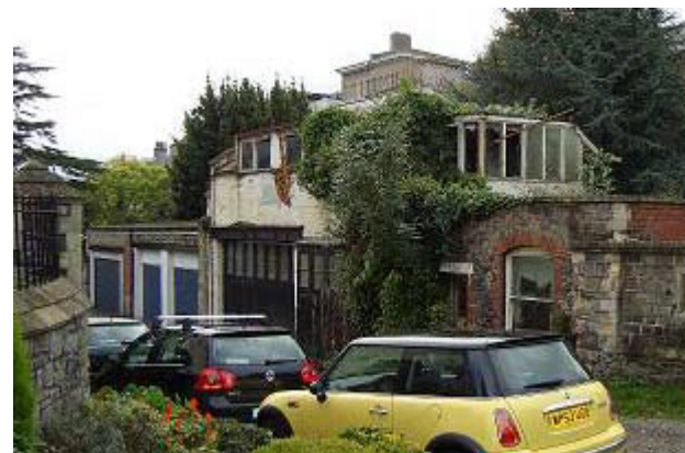
Figure 133: Traditional garage has been left to rot and overgrown with vines. The negative impact is on the character of this mews street which feels neglected and on the traditional garages that are worthy of retention and sympathetic restoration
