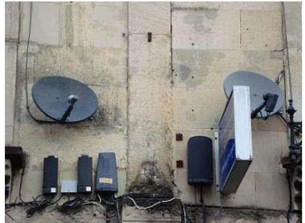
Figure 134: Satellite dishes on the sides of listed buildings are not acceptable. Unauthorised dishes can be enforced against and the owners required to remove them
