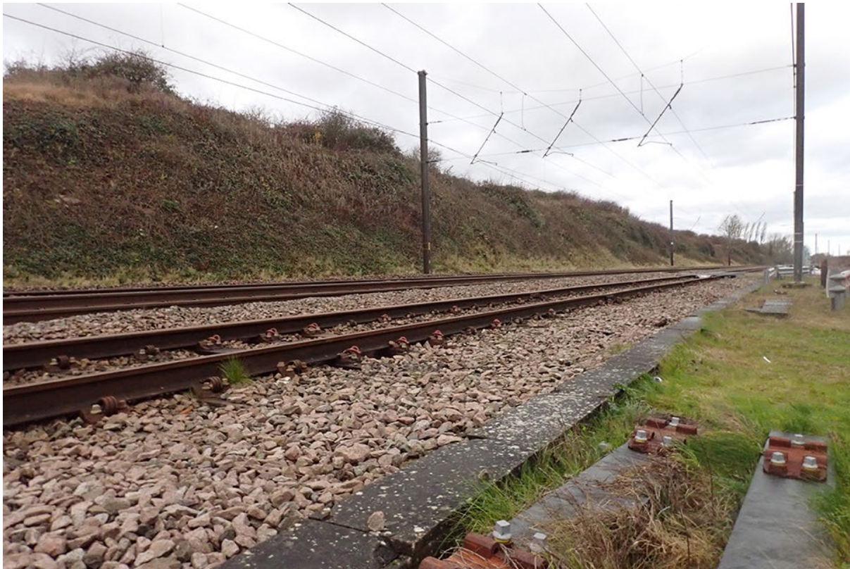
Road-rail vehicle access point at Ponton Yard near Highdyke, looking north towards Grantham.
