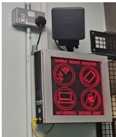
Figure 1.1: Picture of a Wall hound device
