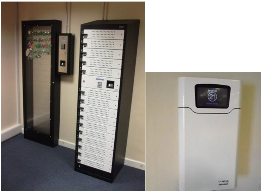
Figure 5.1: Laptop lockers using Electronic Key Management System
