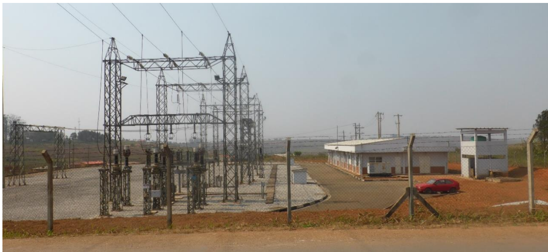
Figure 17 – Negage Substation Current Status
