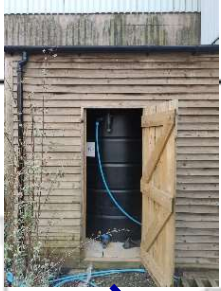
6,000l water storage tank
