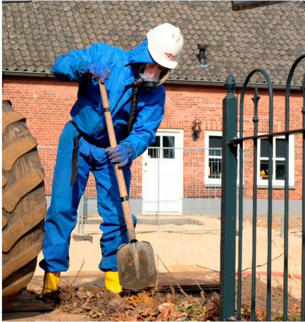
Visual detection of asbestos during remediation | NTP
