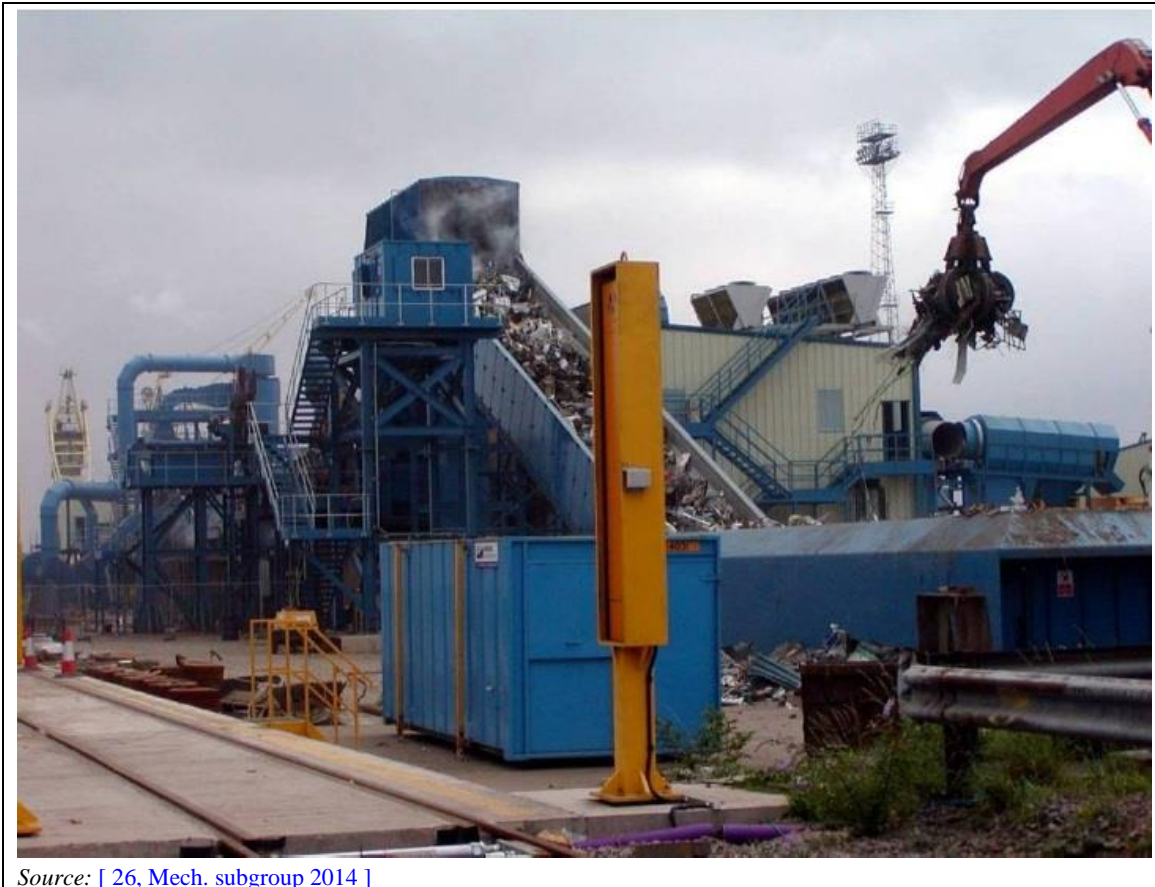
Figure 3.4: A typical EU mixed scrap shredder plant
