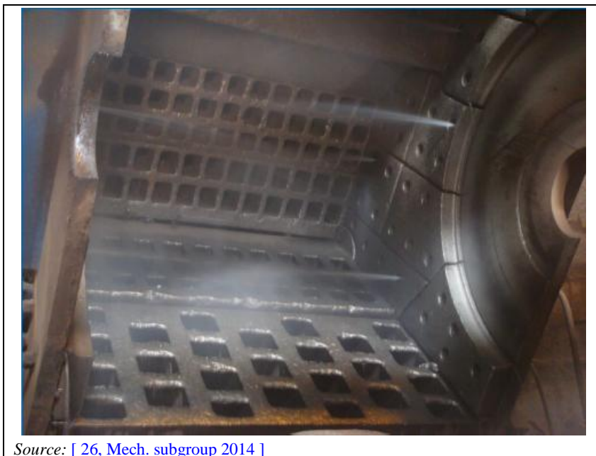
Figure 3.18: Water injection into the shredder mill
