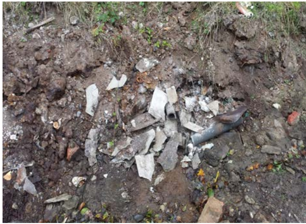
Photo courtesy of Hydrock. Plate 19. Degraded asbestos insulating board (AIB) on surface of made ground.
