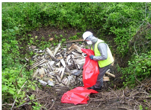
Photo courtesy of VertaseFLI. Plate 5. Collecting fly-tipped broken-up but intact fragments of asbestos cement sheeting waste.
