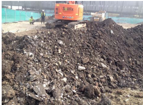
Photo courtesy of Soilfix Limited. Plate 9. Example of weathered asbestos cement debris in excavated made ground.
