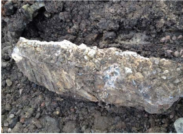
Photo courtesy of Soilfix Limited. Plate 7. Example of asbestos cement shuttering to underside of concrete slab.
