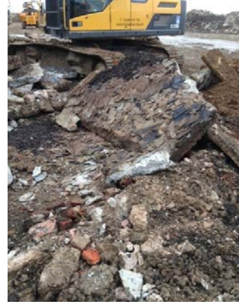
Photo courtesy of Soilfix Limited. Plate 8. Extreme example of intact asbestos cement debris to underside of concrete slab.
