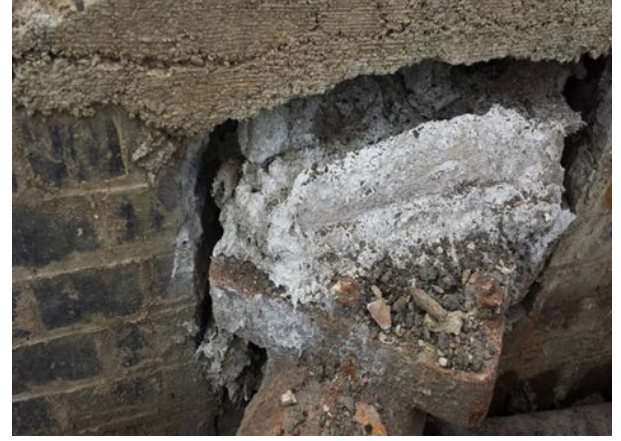
Photo courtesy of Hydrock. Plate 32. Highly degraded/disaggregated asbestos insulation on pipe in underground duct.
