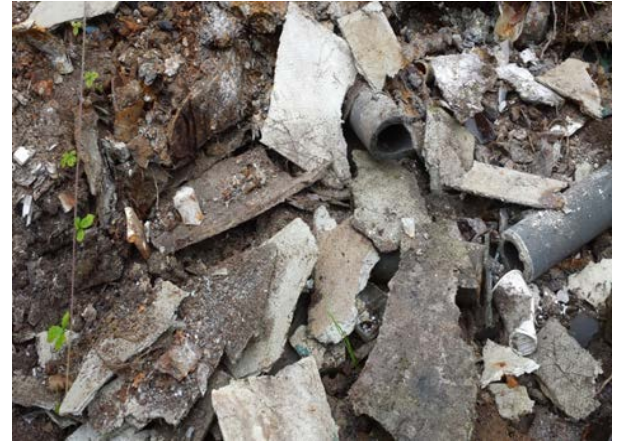
Photo courtesy of Hydrock. Plate 20. Close-up of degraded AIB on surface of made ground.
