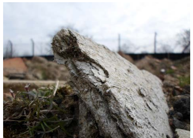
Photo courtesy of Hydrock. Plate 22. Close-up of degraded AIB/fibrous board on surface of made ground.
