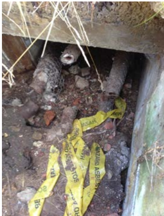
Photo courtesy of Soilfix Limited. Plate 27. Close-up of residual 'original form' asbestos thermal insulation on pipes in underground duct.
