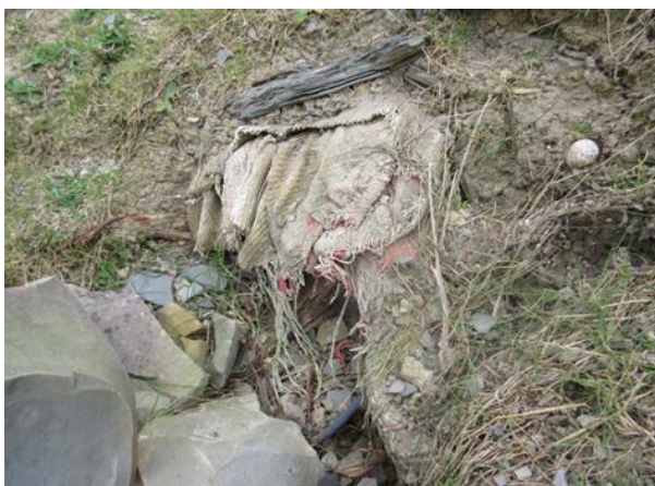
Photo courtesy of Hydrock. Plate 17. Weathered asbestos textile exposed on surface of made ground.
