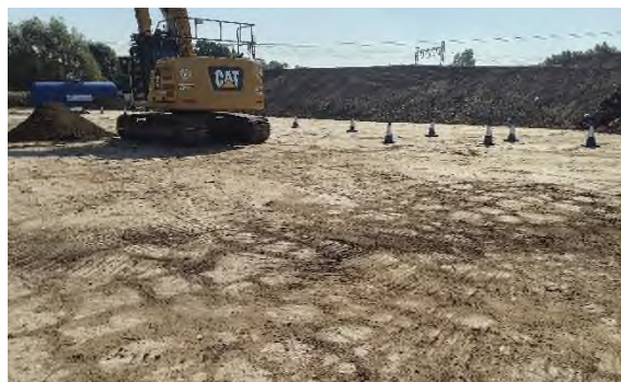
Photograph 6 – 04/09/23 Dust/debris to slab for sampling B
