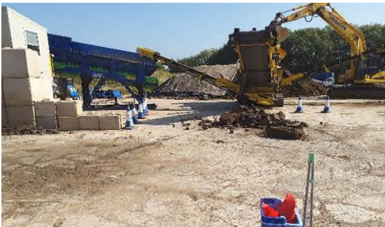
Photograph 5 – 04/09/23 Dust/debris to slab for sampling A
