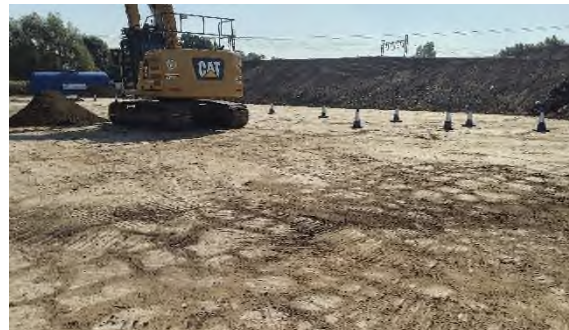
Photograph 6 – 04/09/23 Dust/debris to slab for sampling B
