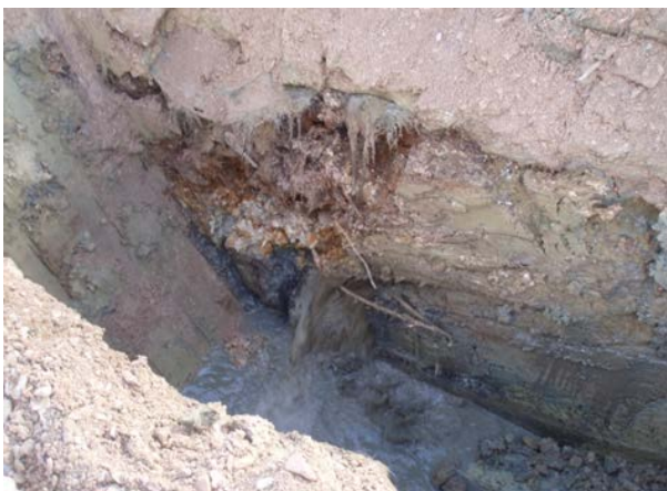
Photo courtesy of Hydrock. Plate 35. Highly degraded/disaggregated asbestos insulation/fibrous debris in excavated made ground.
