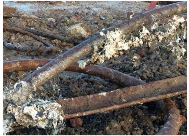
Photo courtesy of Soilfix Limited. Plate 26. Close-up of residual 'original form' asbestos thermal insulation on pipe.
