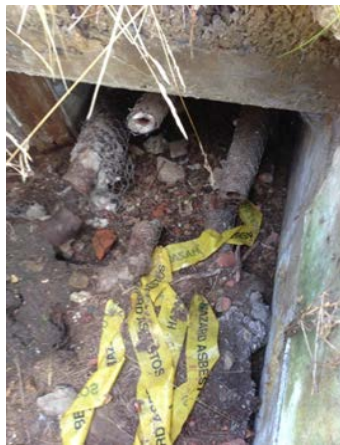
Photo courtesy of Soilfix Limited. Plate 27. Close-up of residual 'original form' asbestos thermal insulation on pipes in underground duct.
