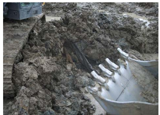
Photo courtesy of Hydrock. Plate 18. Weathered asbestos textile blanket in excavated made ground.
