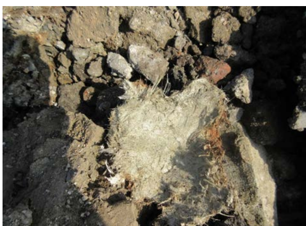
Photo courtesy of Hydrock. Plate 23. Highly degraded/disaggregated AIB/fibrous board in excavated made ground.
