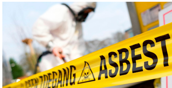
Signing of an asbestos impacted area | NTP
