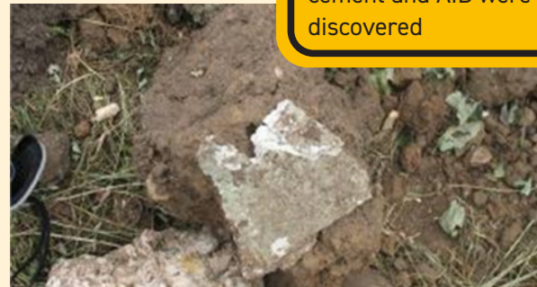
Asbestos finds | Ramboll
