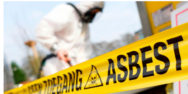
Signing of an asbestos impacted area | NTP
