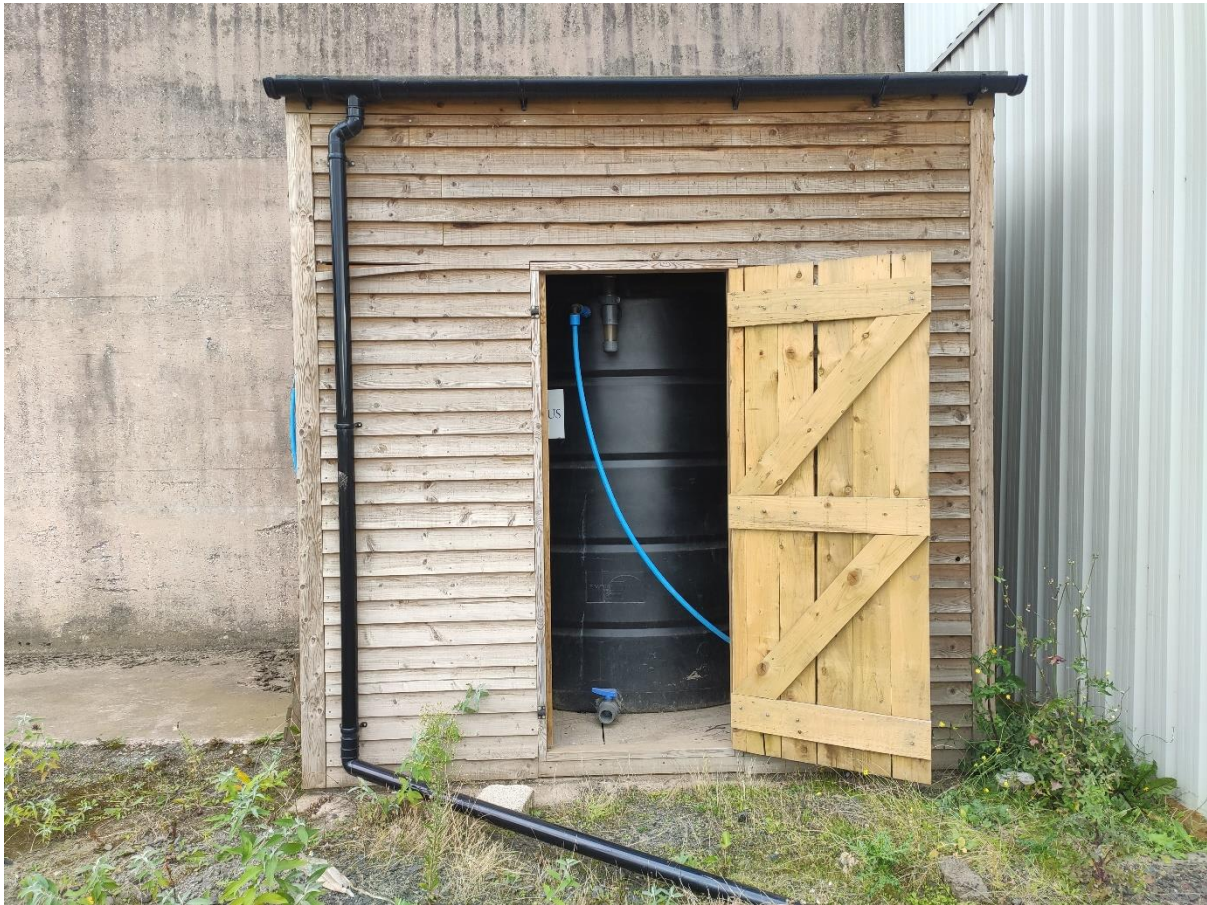
Figure 3. 6m 3 potable water storage tank inside locked enclosure
