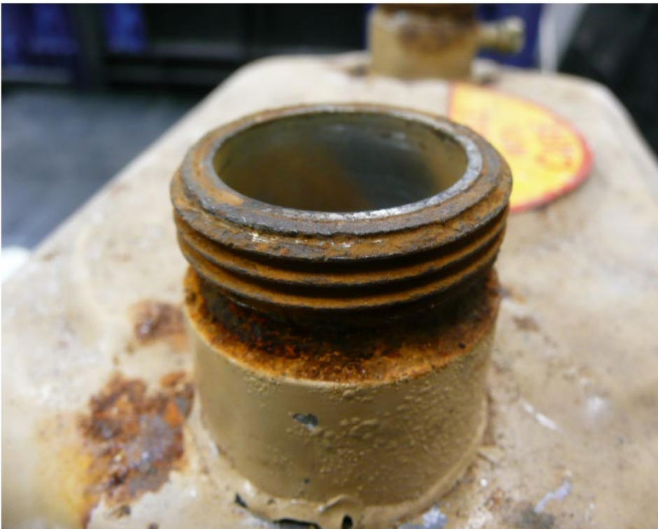
Gas meter – High level of rust on boss
