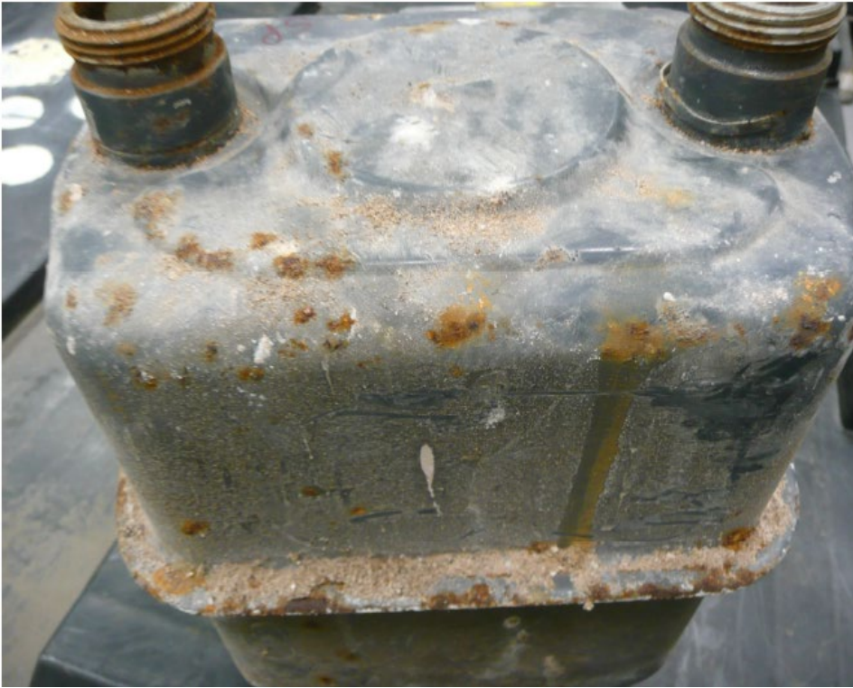
Gas meter – Low level of rust on body
