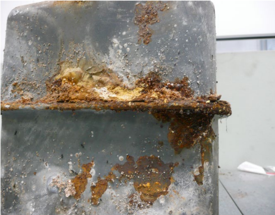
Gas meter – High level of rust on body
