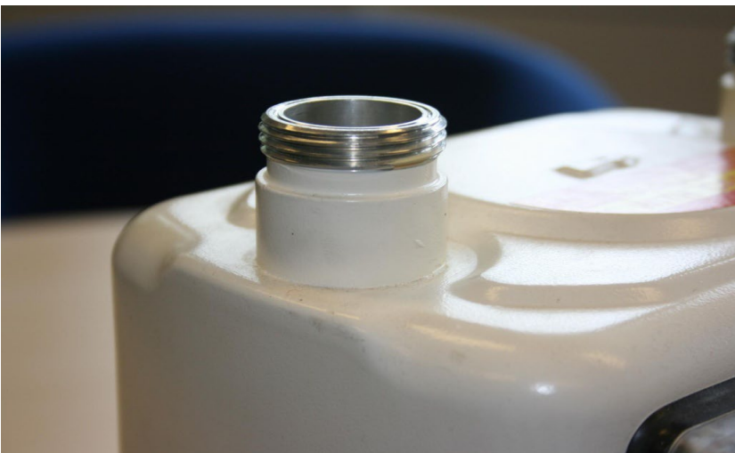
Gas meter – No rust over meter boss
