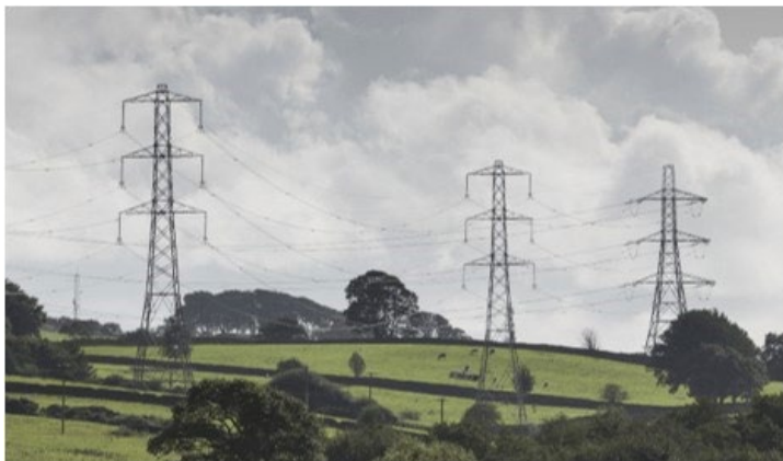
Lattice pylon image courtesy of National Grid
