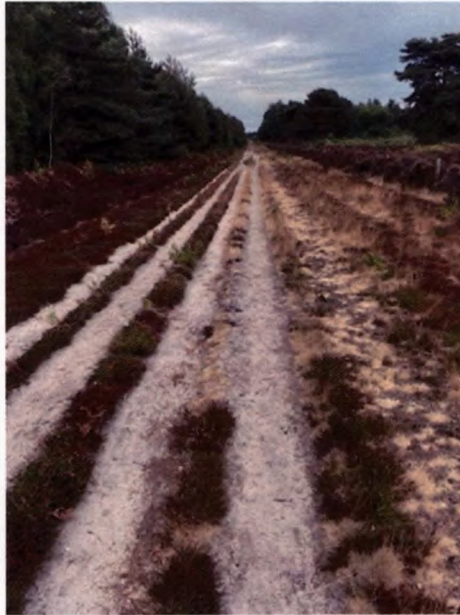
Figure 1.3.2 - The Green Mile at point of collapse
