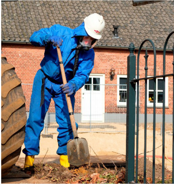
Visual detection of asbestos during remediation | NTP
