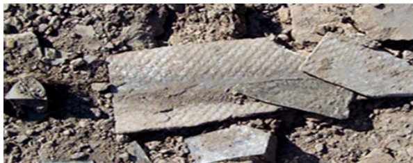
Asbestos cement fragments in soil | AECOM
