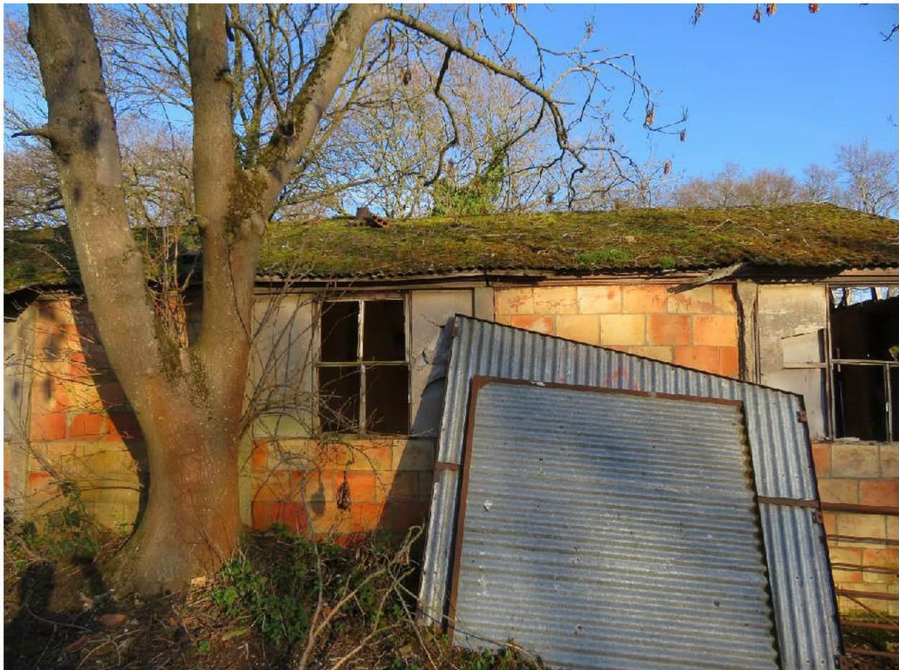
Photograph 20: Local damage to structure from self-sown tree
