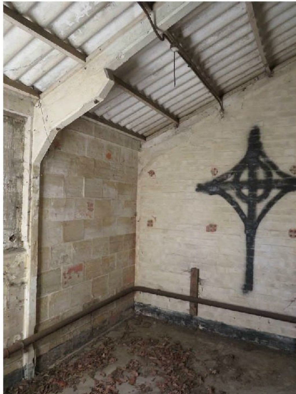
Photograph 2: Pre-cast concrete post with integral elbow and pre-cast frame rafter above
