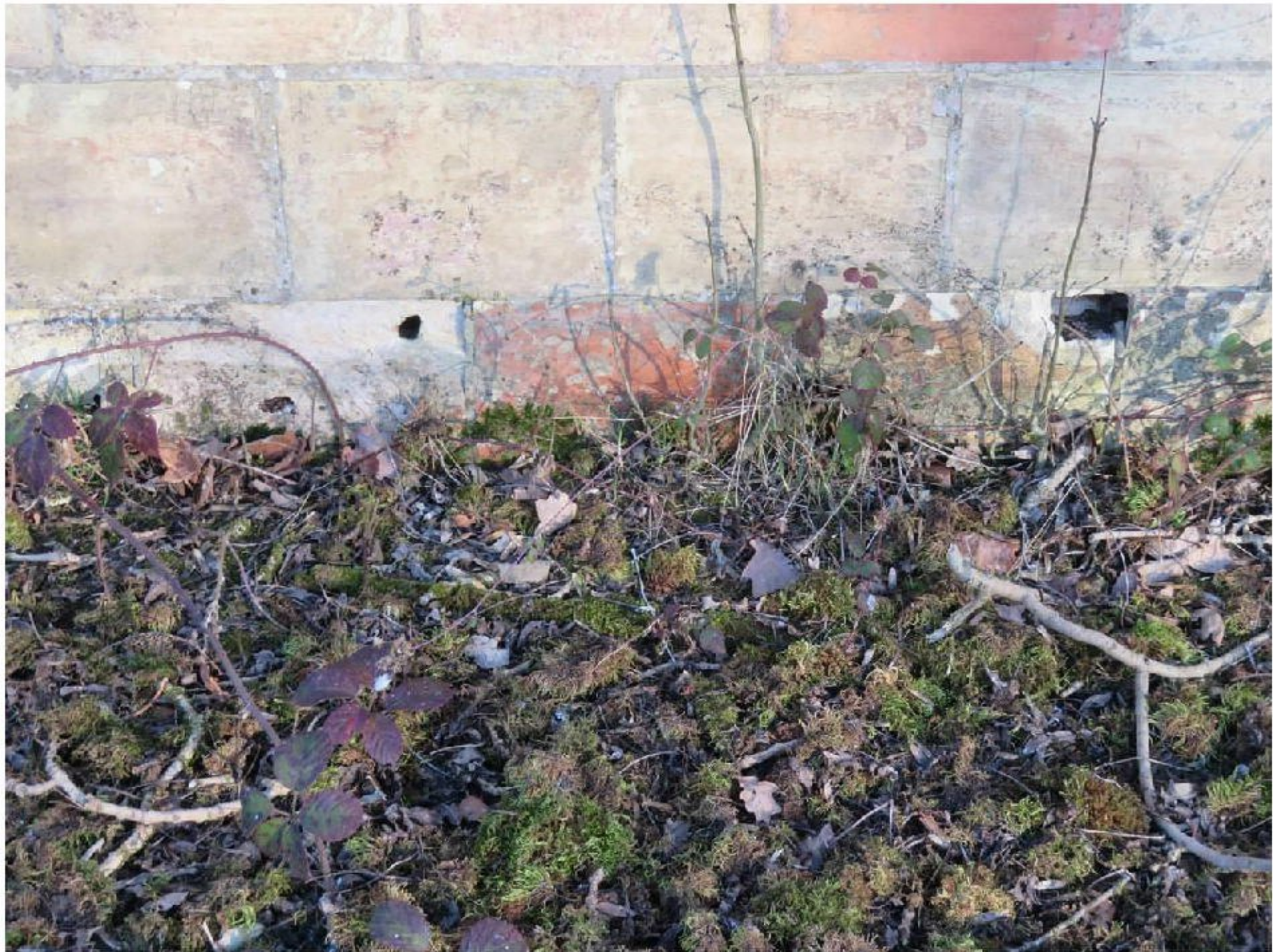
Photograph 21: Locally damaged hollow blocks due to damp
