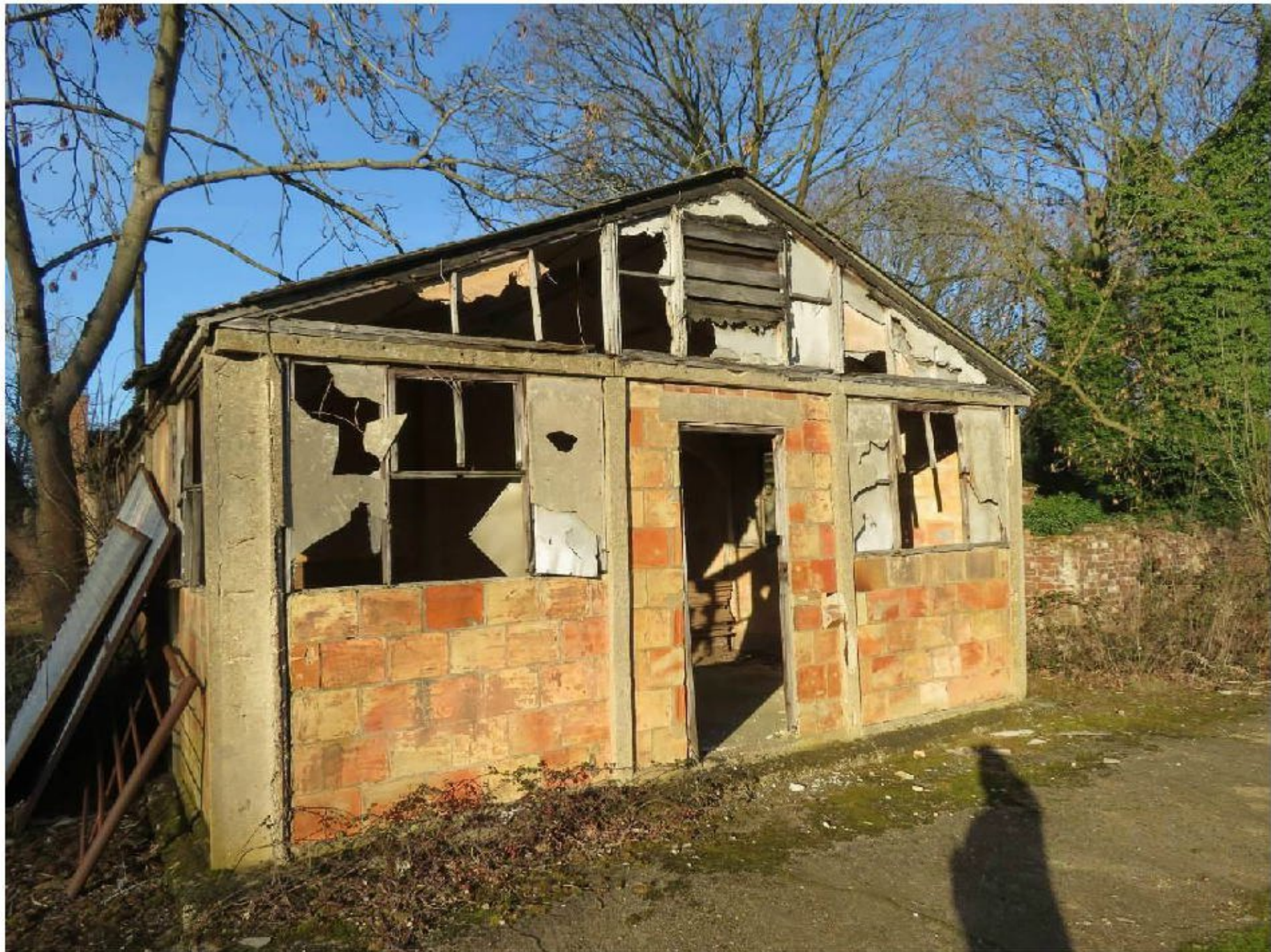
Photograph 5: Typical gable with tie at eaves level in three sections and secondary posts
