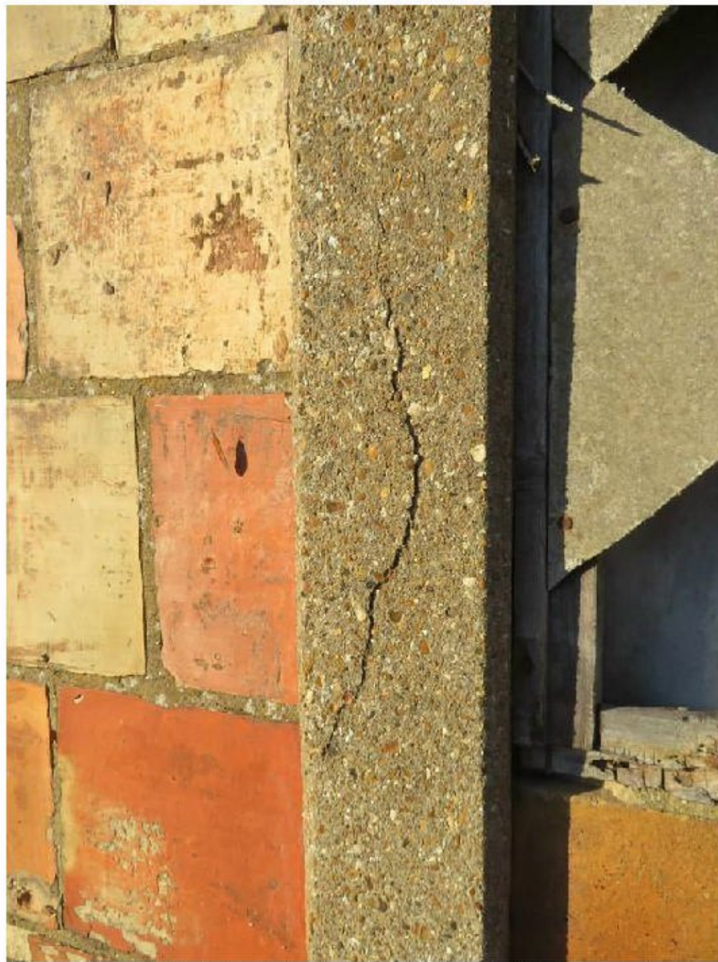
Photograph 19: Cracking to post suggesting reinforcement corroded below
