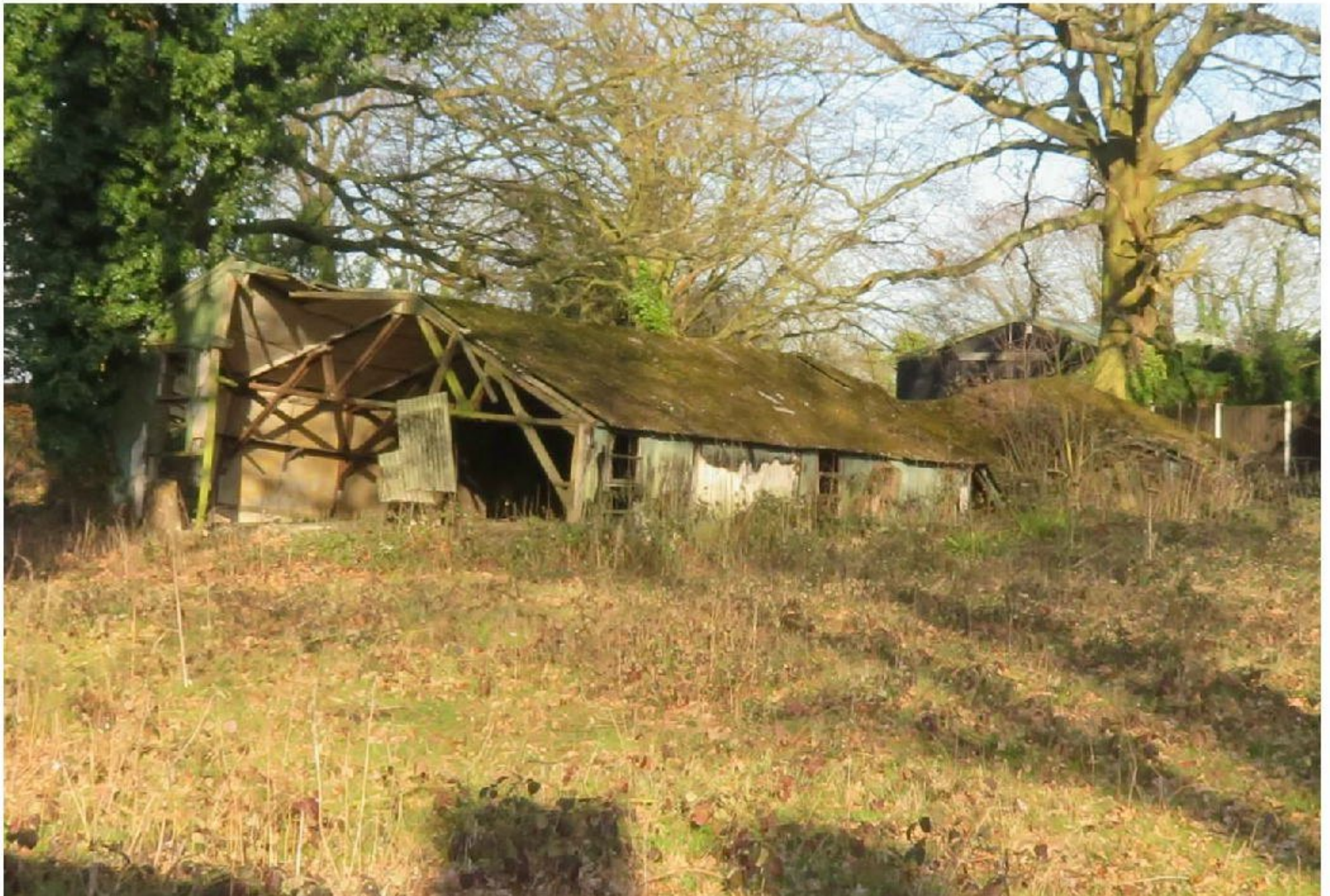
Photograph 14: Building 8 with part collapsed walls
