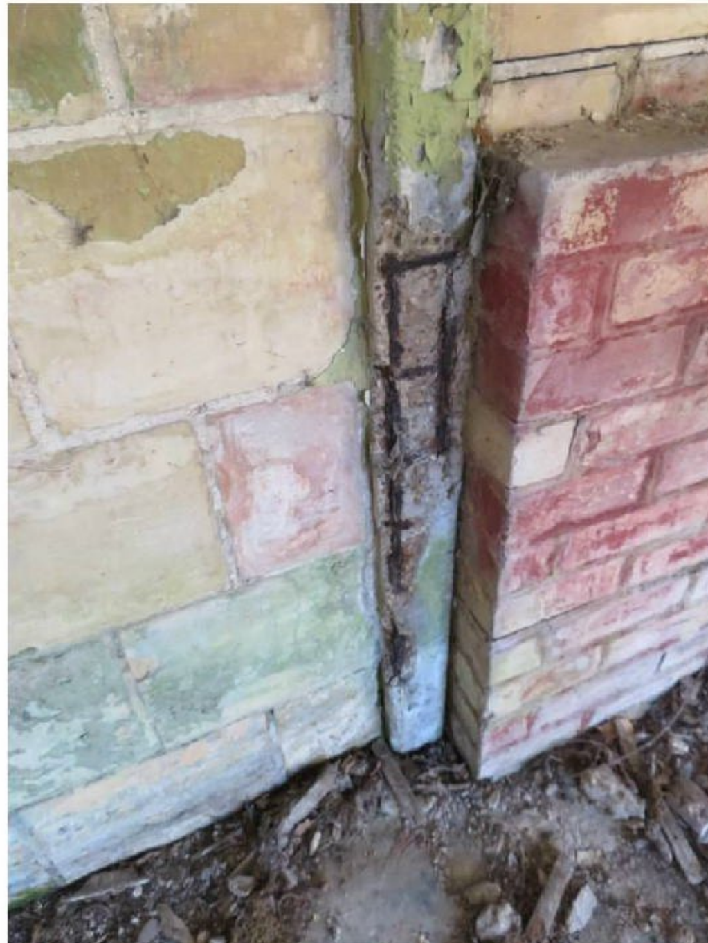
Photograph 18: Reinforcement corrosion and concrete cover lost to post
