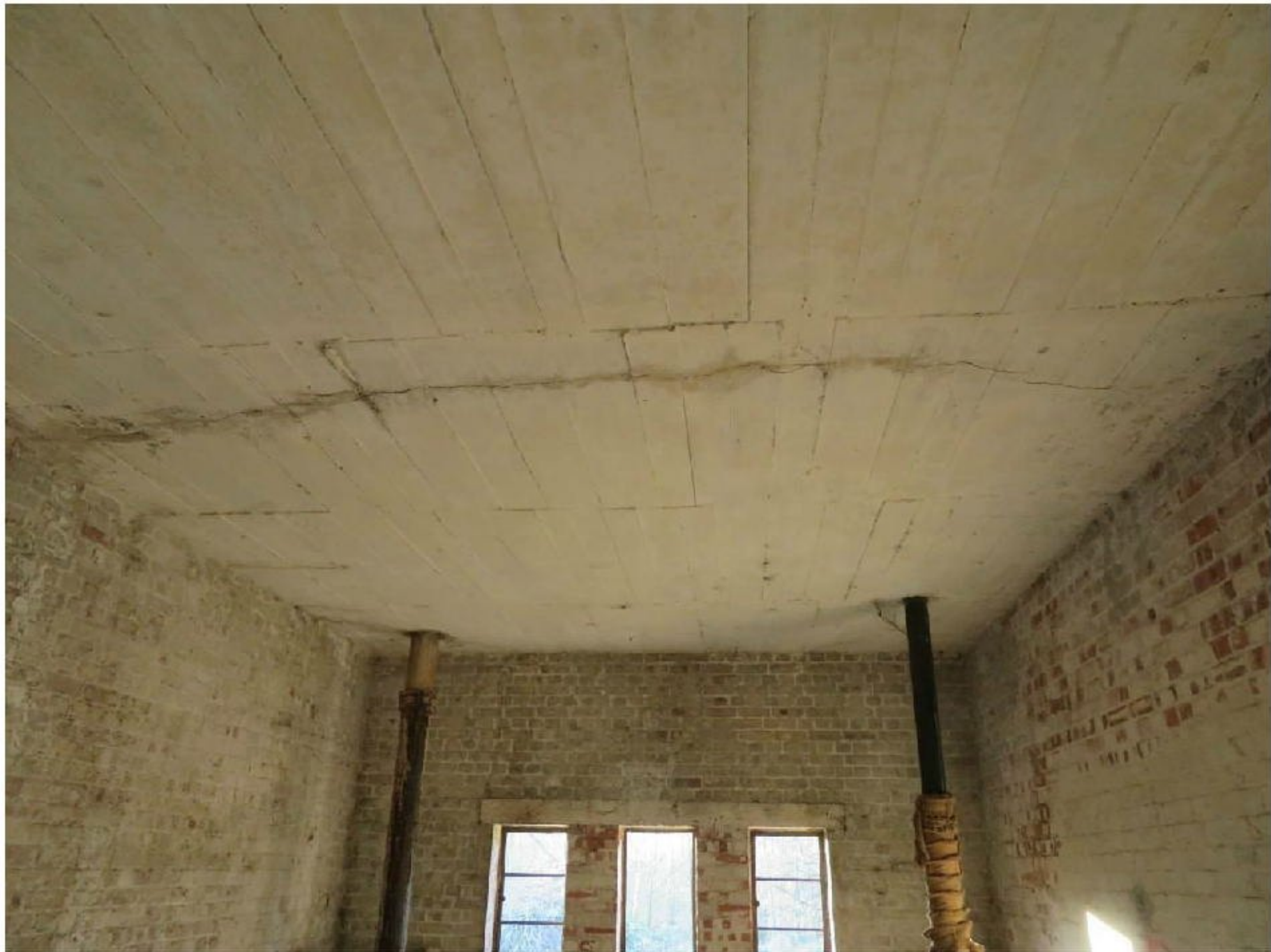
Photograph 27: Internal concrete slab with central crack
