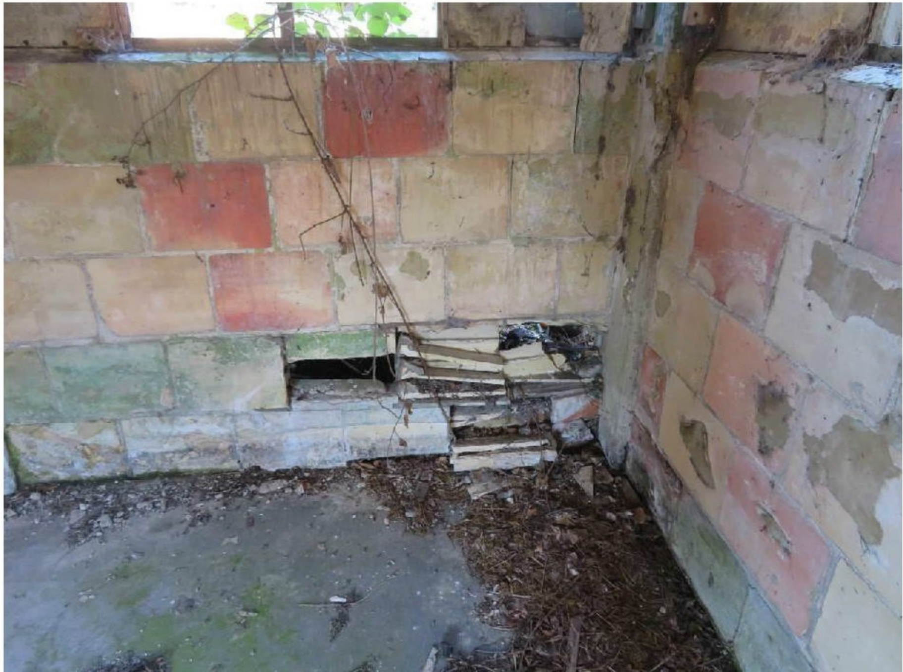
Photograph 22: Locally damaged blocks due to high external ground levels
