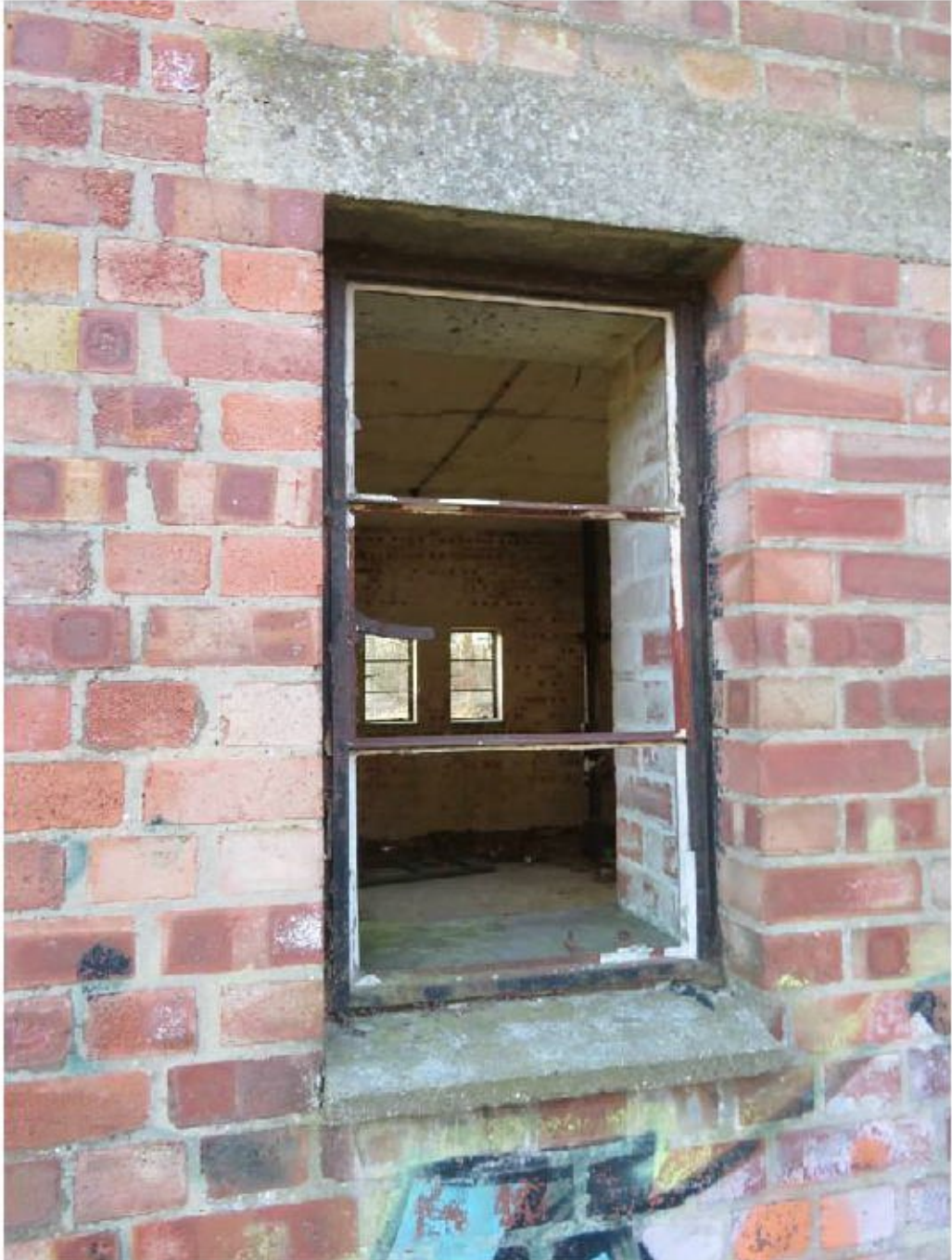
Photograph 25: Crittal window to Water Tower
